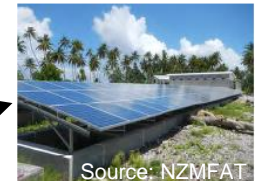
Tokelau PV, Lead Acid Batteries, control
