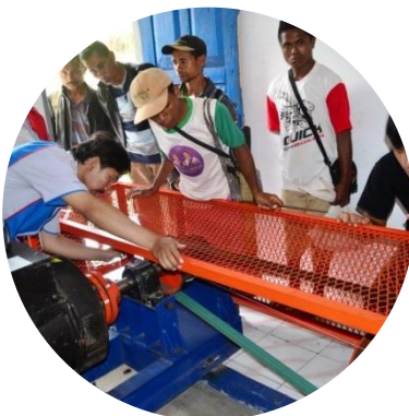
TECHNICAL REVIEW Compatibility of components Verification of performance Quality of installation
