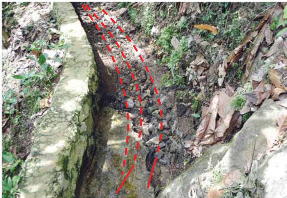
Broken channel invert caused by erosion and sliding
