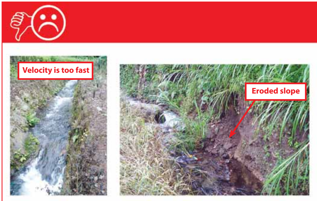
Earth channel can erode easily when velocity is too high
