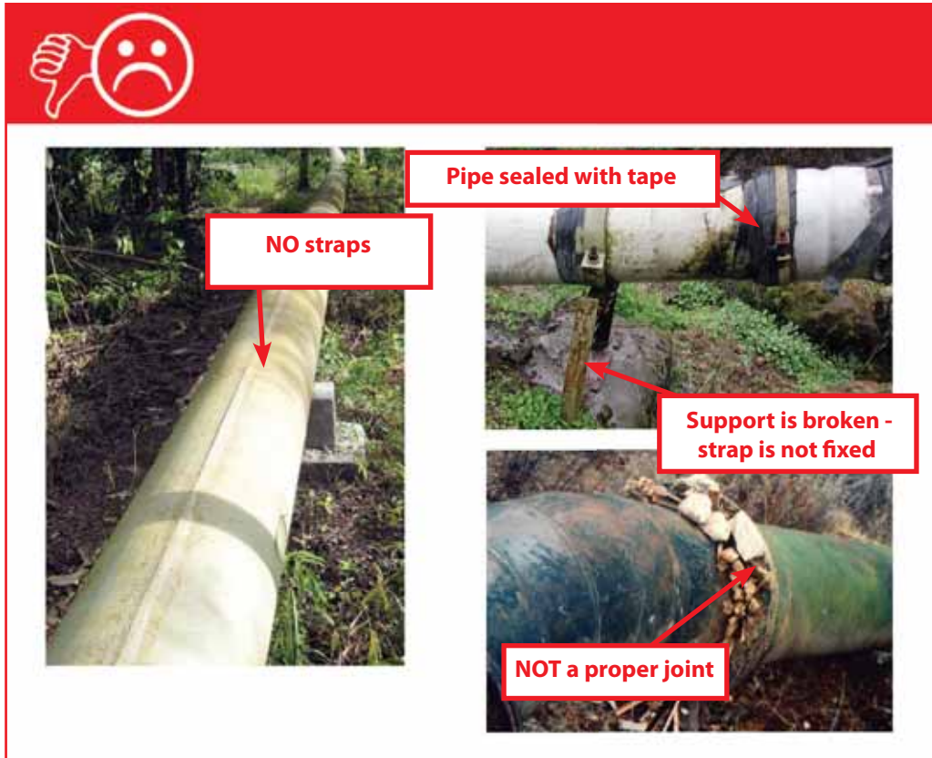
Several examples of poorly installed penstocks
