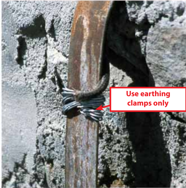
Earthing connection will probably not work
