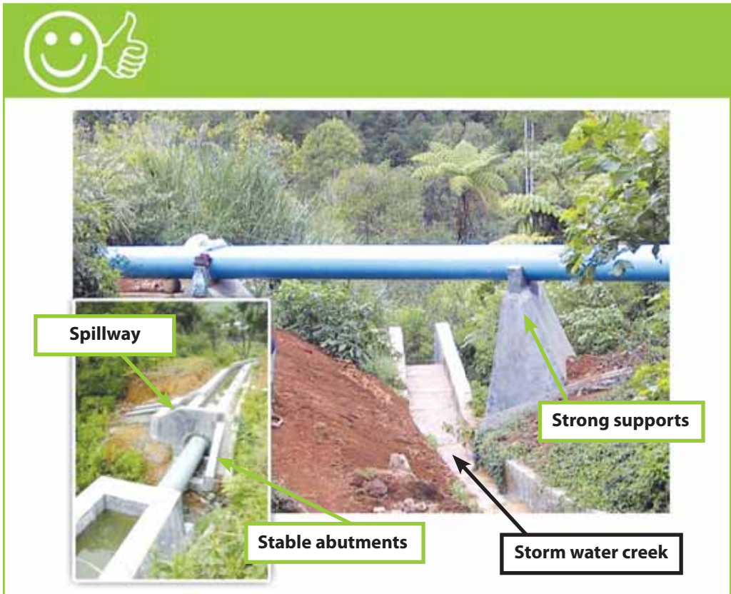
Well-built pipe crossings in a headrace
