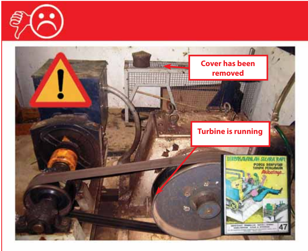
Flywheel and belt are not protected in a cage
