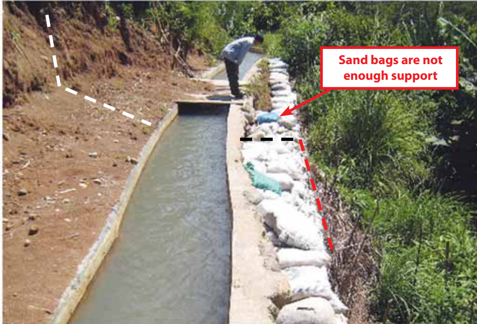
Headrace channel too close to a steep slope
