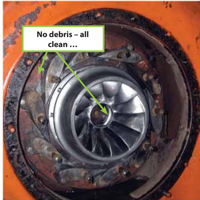
A turbine in good condition – thanks to a functional sand trap and trash rack
