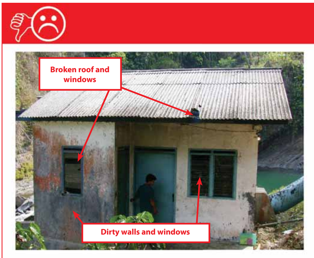
This power house is NOT a safe place for valuable equipment
