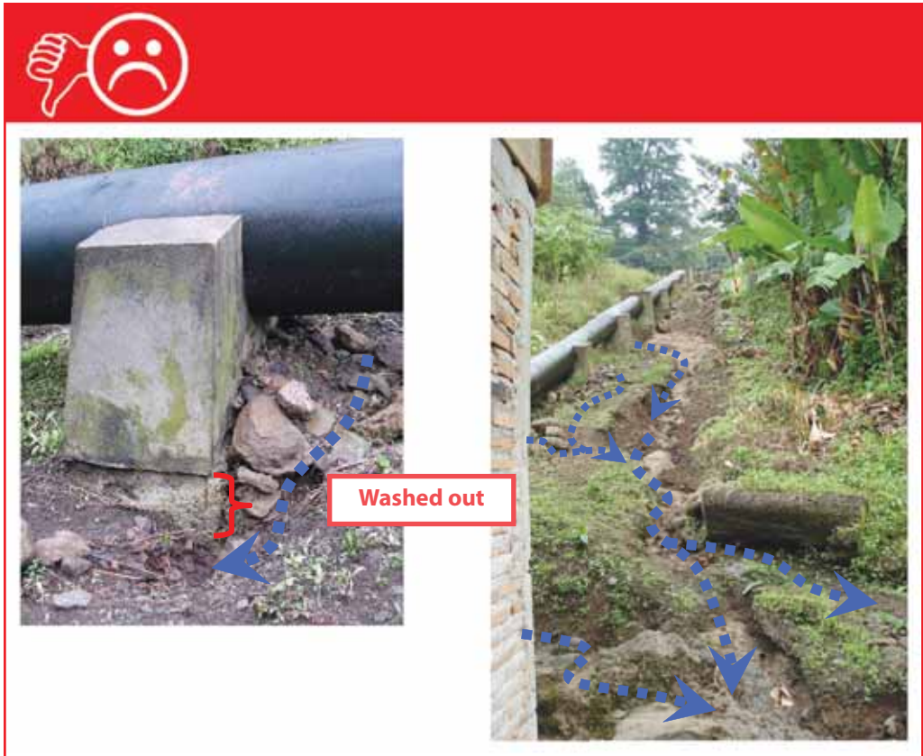
Dealing with surface water; here: uncontrolled water flow
