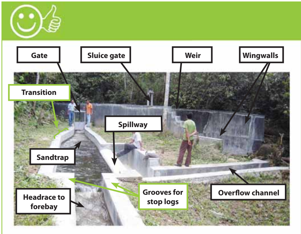
This picture shows all main elements of a well designed water intake with sandtrap
