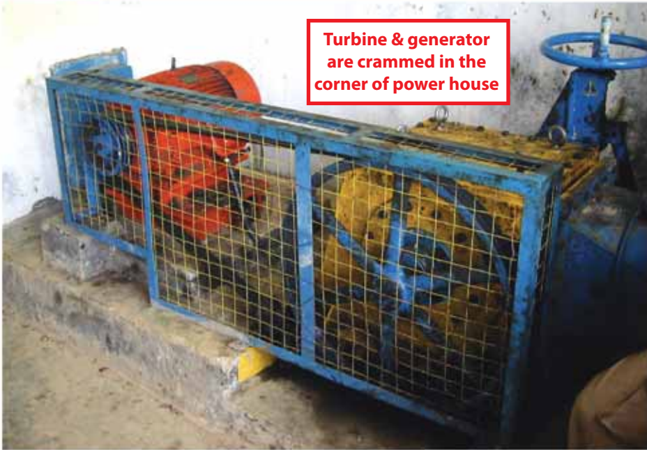
Main equipment is too close to walls
