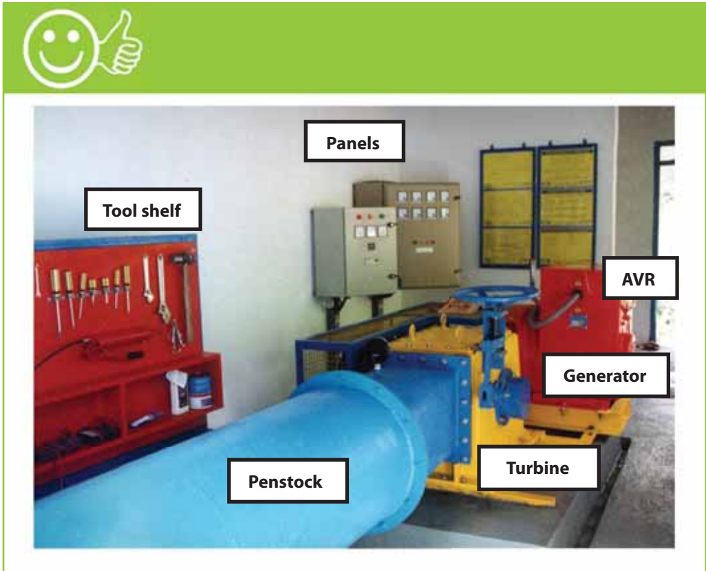
All equipment is well arranged, clean and well maintained
