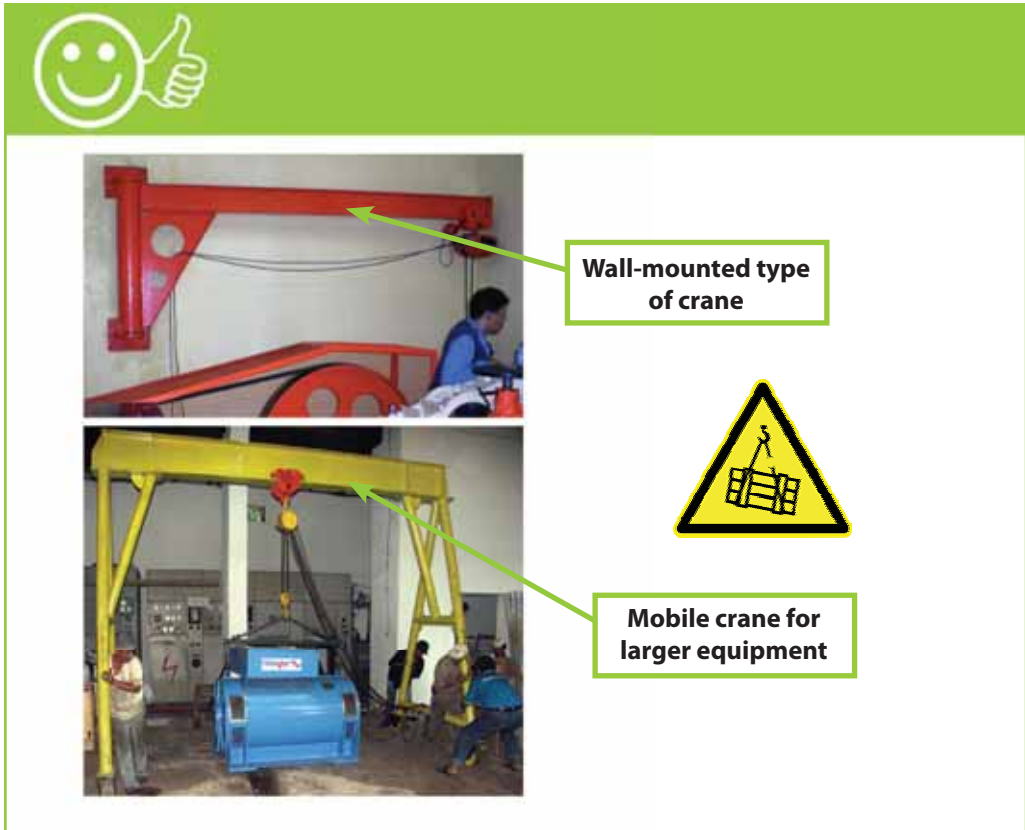
Two types of lifting equipment for heavy loads in larger power houses
