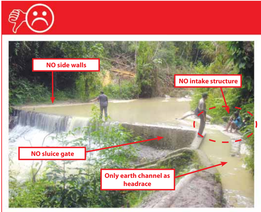
Most elements of a proper weir and intake structure are missing
