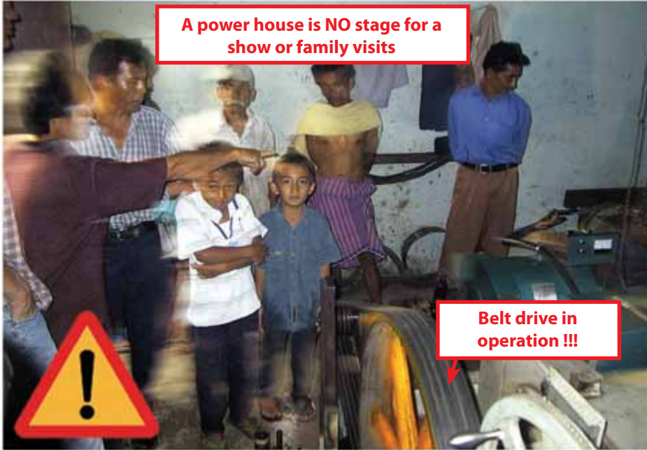
Power house is NO stage for a show or family visits
