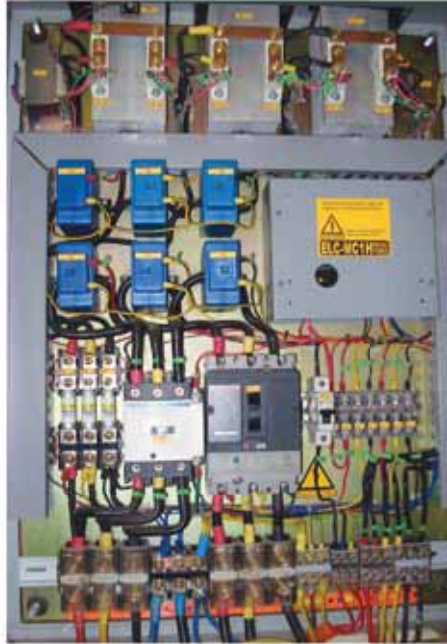
Devices of power and control cubicle
