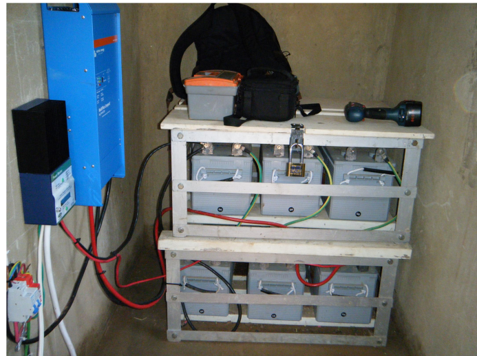
Figure 6.11: Batteries protected in vented battery box
