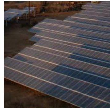
Figure 5.3: Shadow caused by solar PV modules
