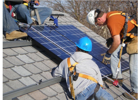
Figure 2.1: Solar PV installers wearing all required PPE – Courtesy: The Solar Planner , www.thesolarplanner.com
