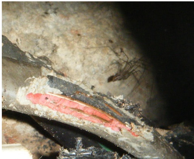
Figure 7.1: Rodent bites on a cable
