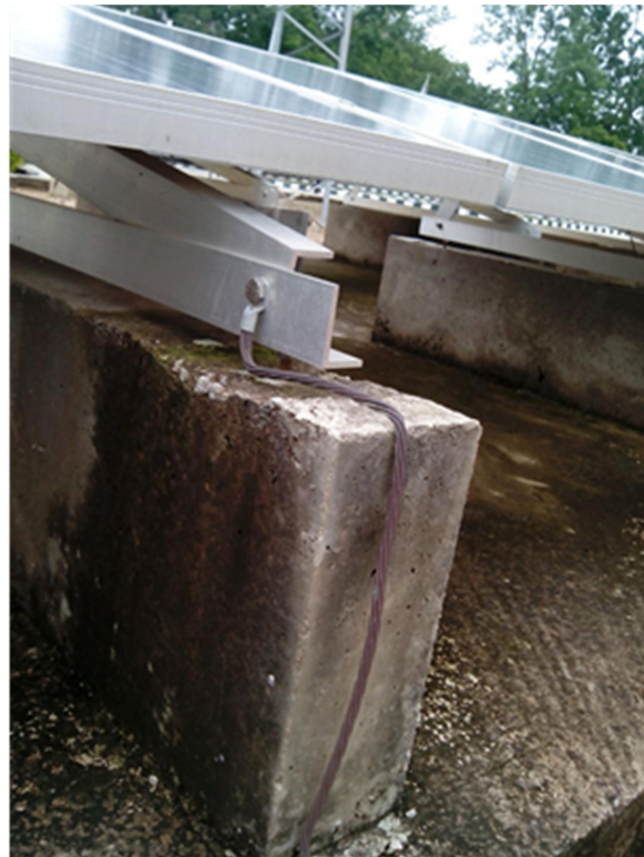
Figure 3.39: Grounded solar array
