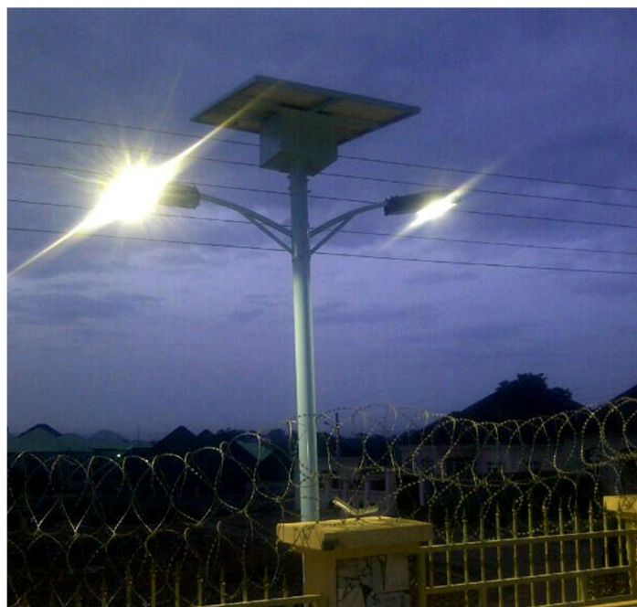
Figure 1.23: Solar street light in Umuahia, Abia State
