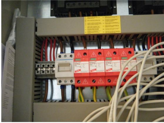
Figure 3.37: DC surge arrestors
