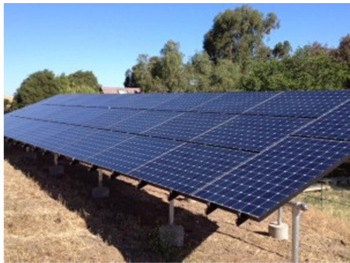
Figure 5.7: Ground-mounted solar PV array – Courtesy: Melissa Van Hoorne, http://blog.solarmicronics.co
