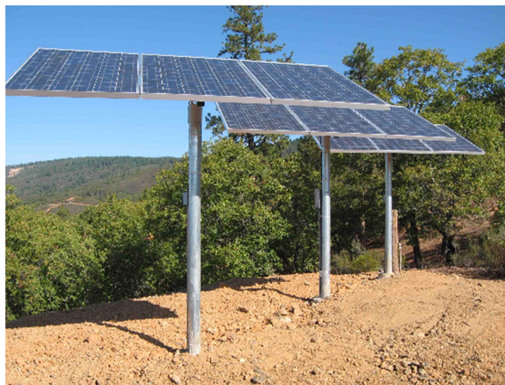
Figure 5.8: Pole-mounted PV array – Courtesy: Accutrack Solar System, www.accutrack.com
