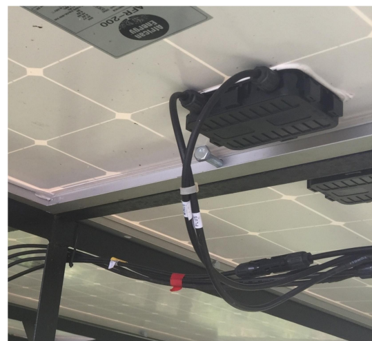
Figure 6.6: Wiring of solar modules with MC4 connectors
