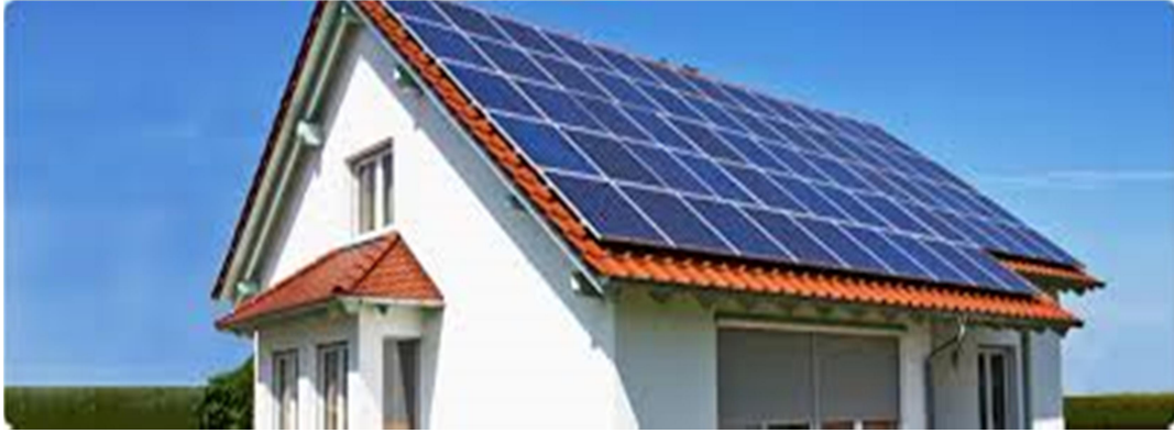
Figure 5.6: Flush-mounted PV modules on a pitched roof
