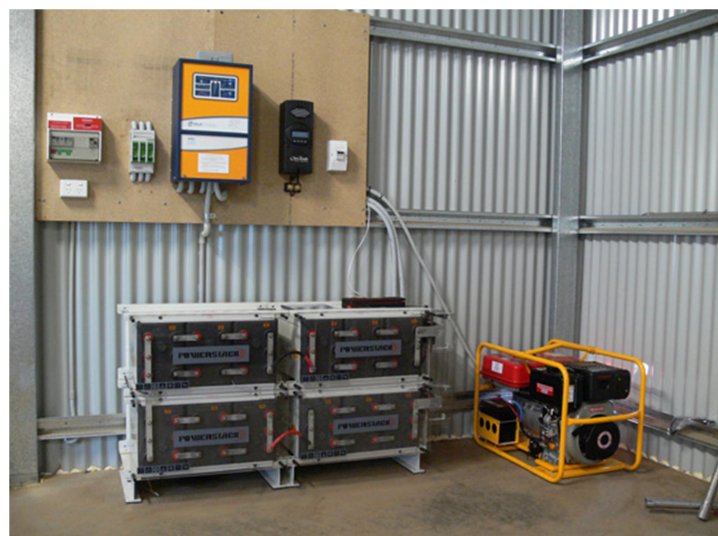
Figure 6.9: 48 V battery bank in a solar hybrid system – Courtesy: www.solarconnections.com.au
