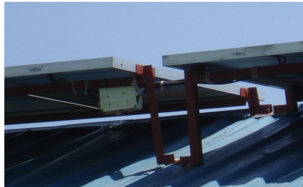
Figure 6.8: Connection of module wires in the junction box
