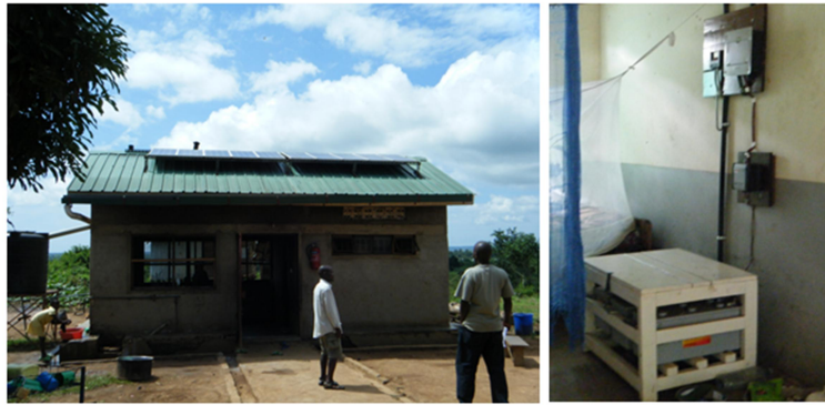
Figure 1.24: Mains supply solar home system with rooftop mounted panels
