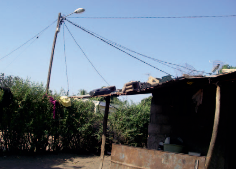
Almost every neighbourhood has public street lighting. But some people mourn that it is often not functioning.
