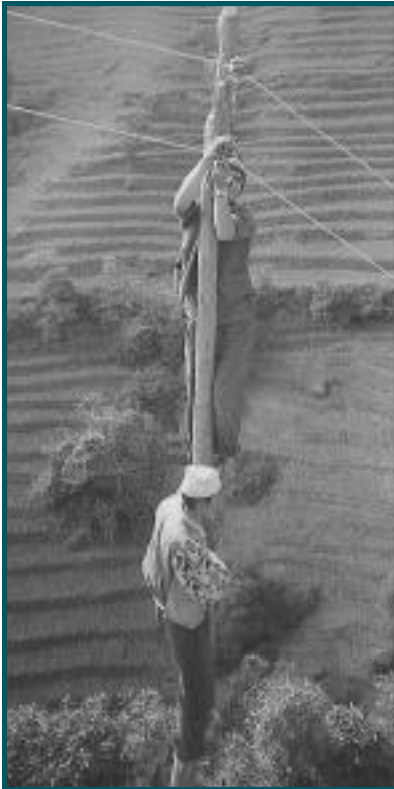
Fixing the cable
