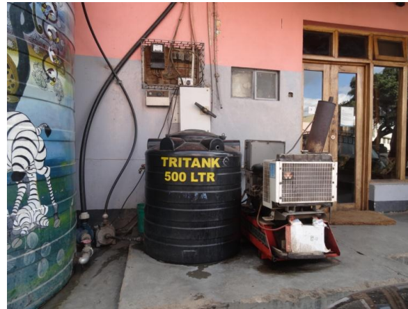
Diesel generator with diesel storage tank – Arusha, Tanzania (Cader, 2015).
