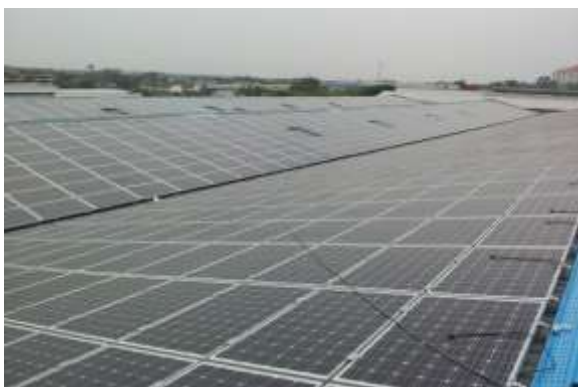
4 MW, Rooftop, Malaysia, 2012
