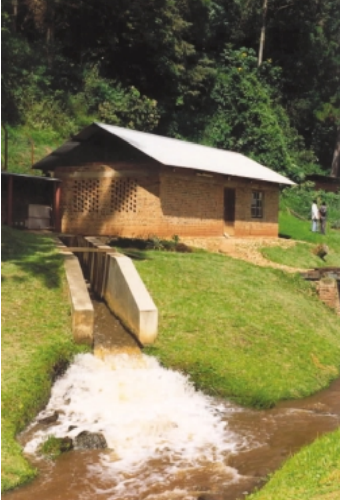
Above: View of the turbine house at Kisiizi hospital in south west Uganda
