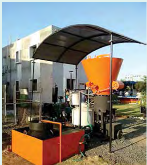
11-kWe Basic, non containerized power generating system.
