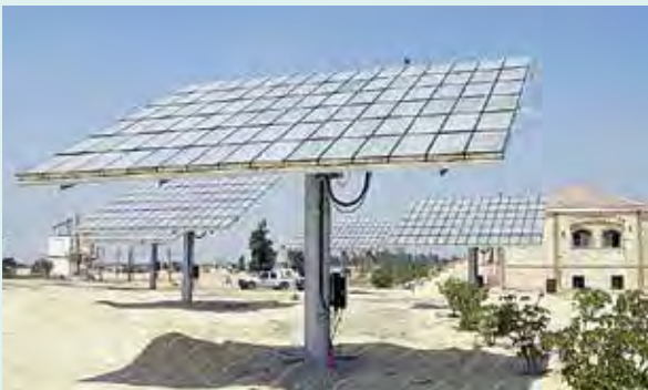
CPV stand-alone system in the Wadi El Natroon, 100 km northwest of Cairo, Egypt.
