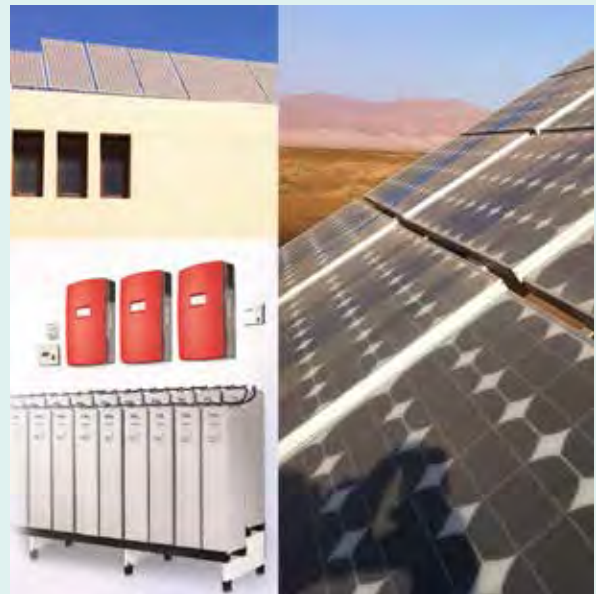
Private home pv off-grid system in Egypt, size: 24 kWp
