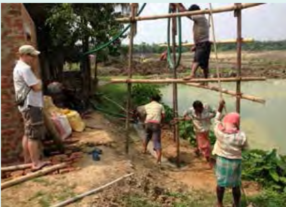
Drilling of bank filtration well in Kalyani in West Bengal, India, SWINGS-project.
