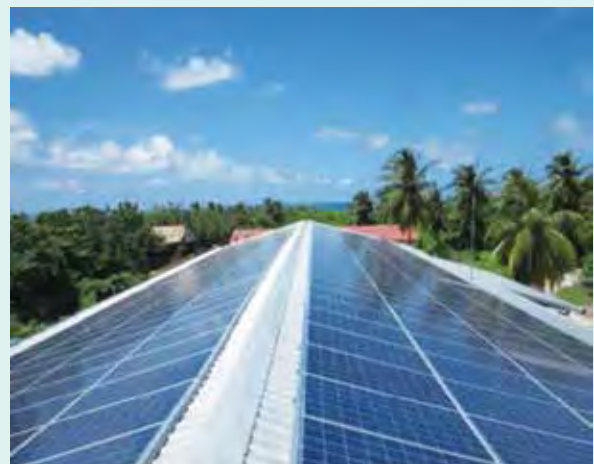
Solar installation on sewerage building on Ungoofaaru Island, Maldives.
