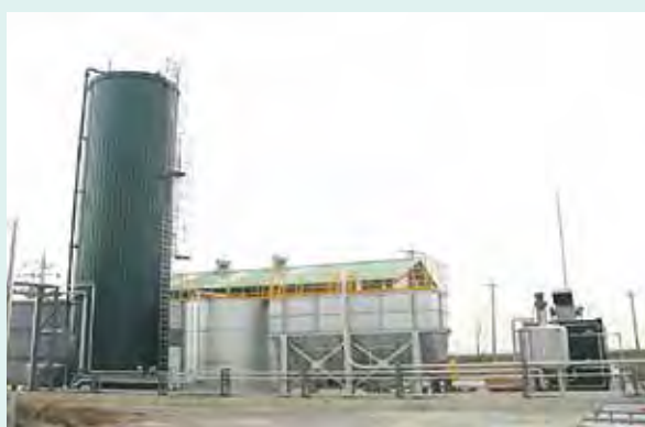
8t/h Food waste biogas plant in South Korea.
