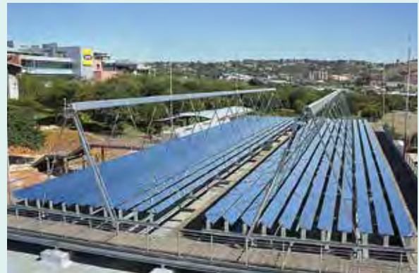
Fresnel Collector (LF 11) serves the district cooling plant of MTN Headquarter in South Africa.
