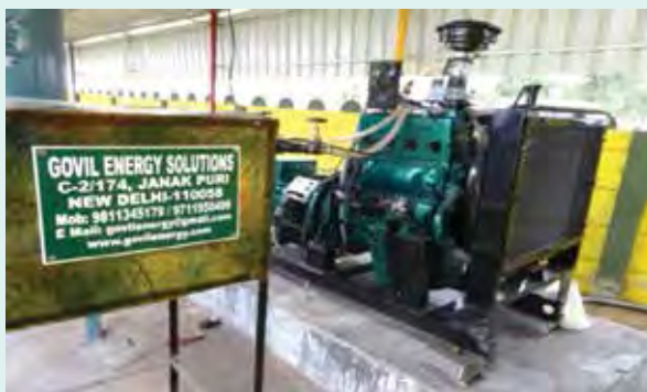
15 KVA biogas generator at Behel India.
