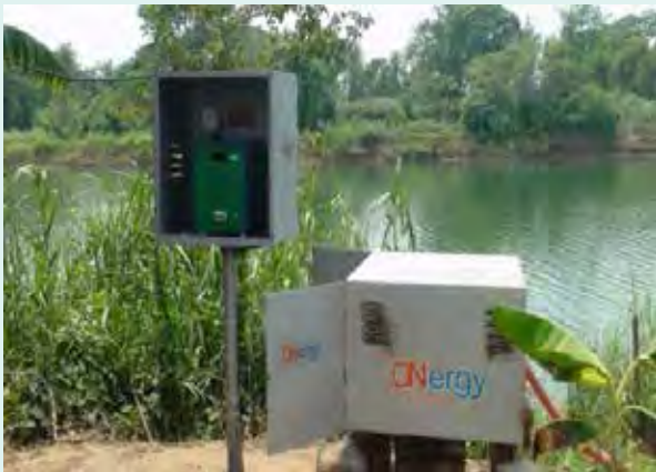
Source, pump set and control unit.
