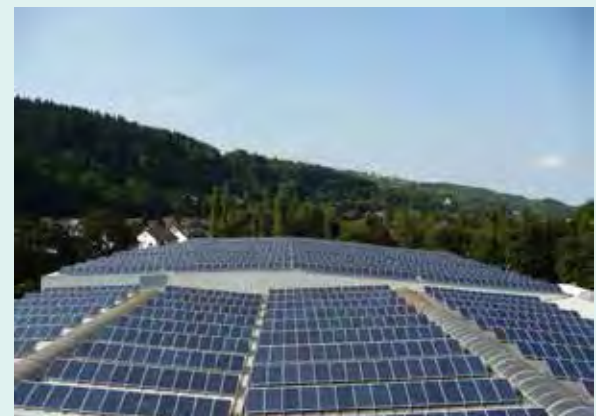
Photovoltaic off-grid installation with high-end solar modules/inverters/batteries, size: 98 kWp.
