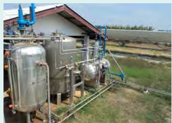
TRESERT - Tri-Generation facility in Thailand generating heat, electricity and cooling using solar energy in combination with biomass.
