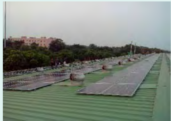
KISS 500 KW solar plant, Odisha.
