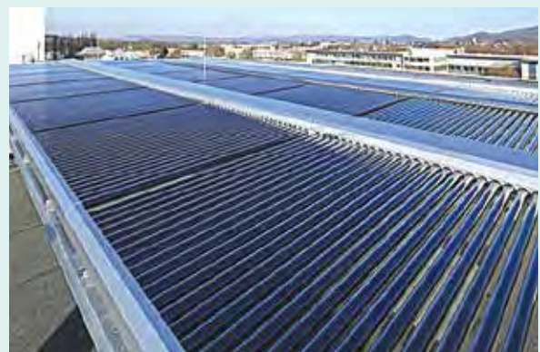
Air-Collector (Sun-Storm) serves a drying process at Pfizer in Germany.
