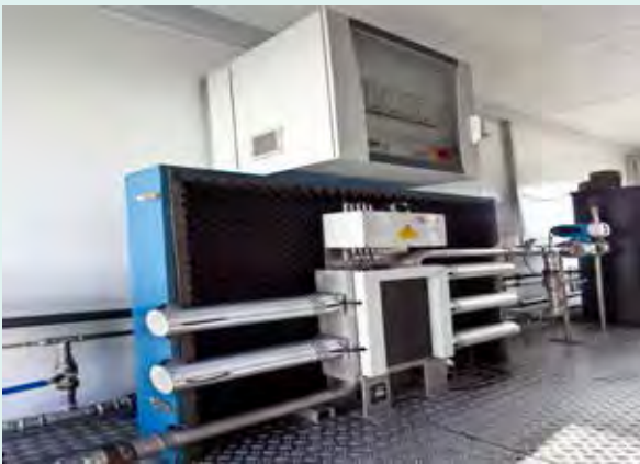
Installation of a high-power ultrasound plug-flow system.
