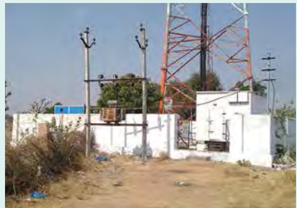
10-kWe Gasifier based power generation system for telecom towers.
