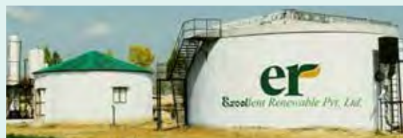
Commercial biogas plant at Abohar, Punjab.
