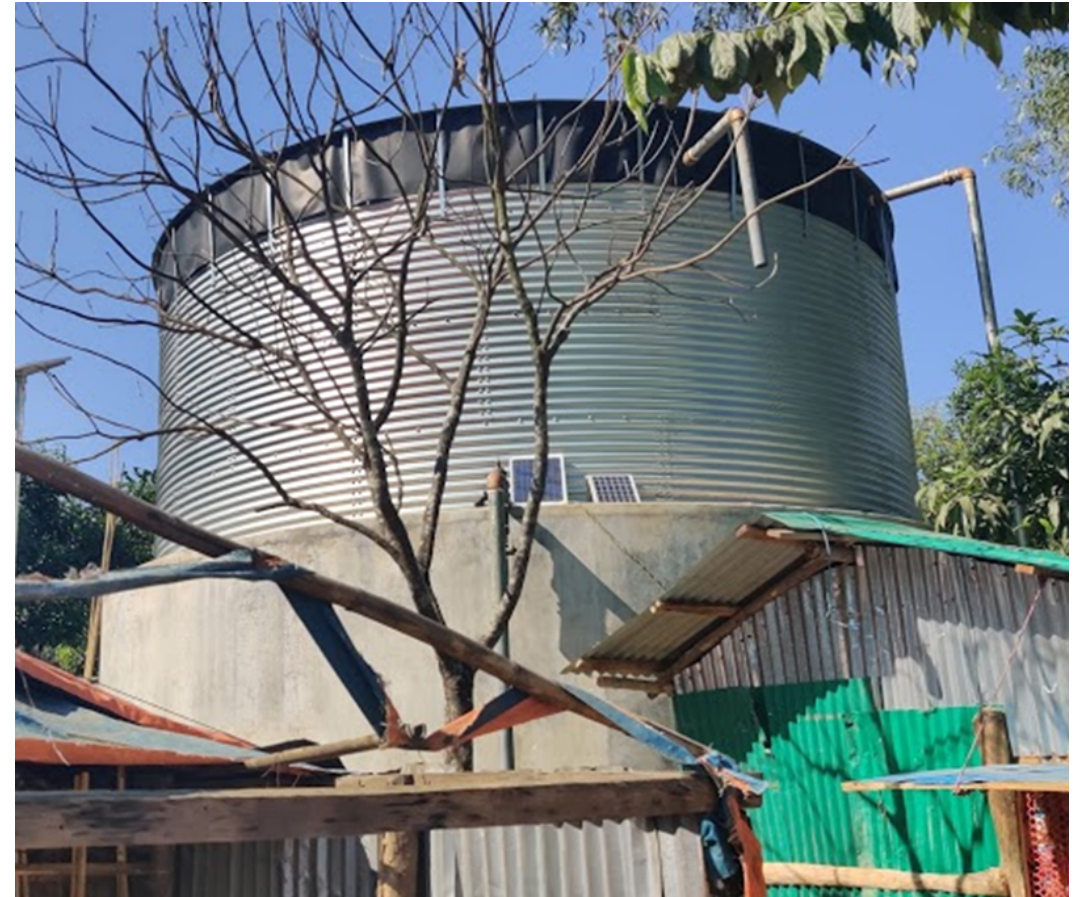
95m3 steel storage tank
