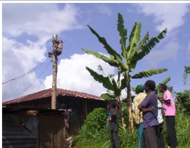
The first house is connected to the generator
