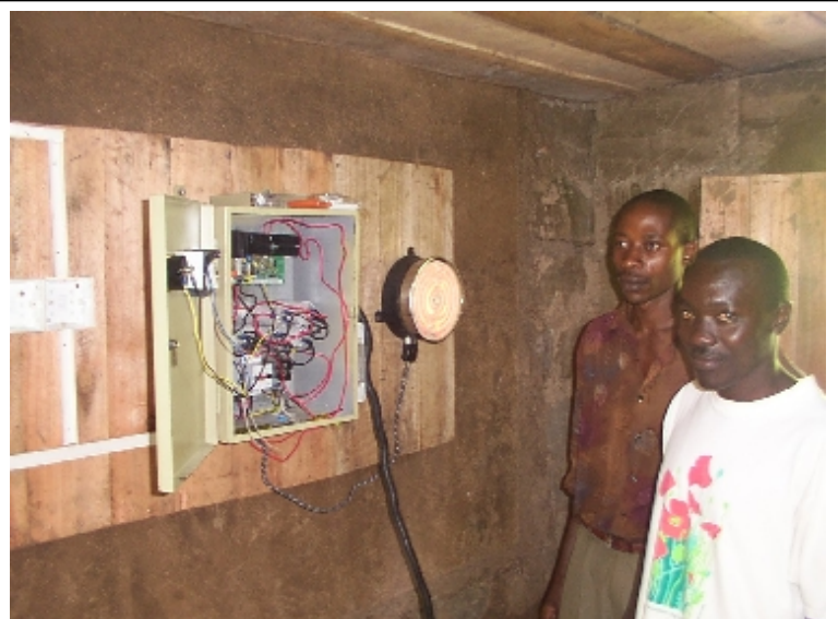
Trained pico hydro installers and operators, Peter Kinyua Mbui and David Kinyua with the IGC enclosure and ballast.
