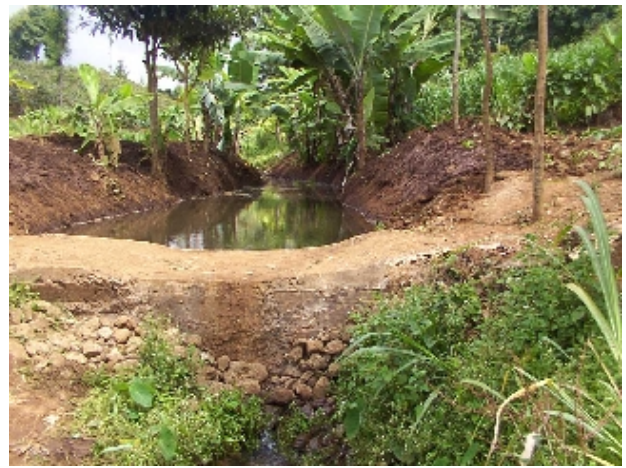
Completed intake with storage pond
