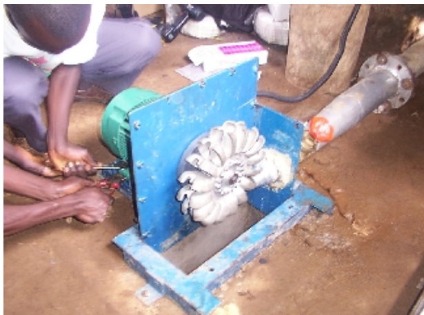
200 p.c.d. Pelton Turbine and Nozzle
