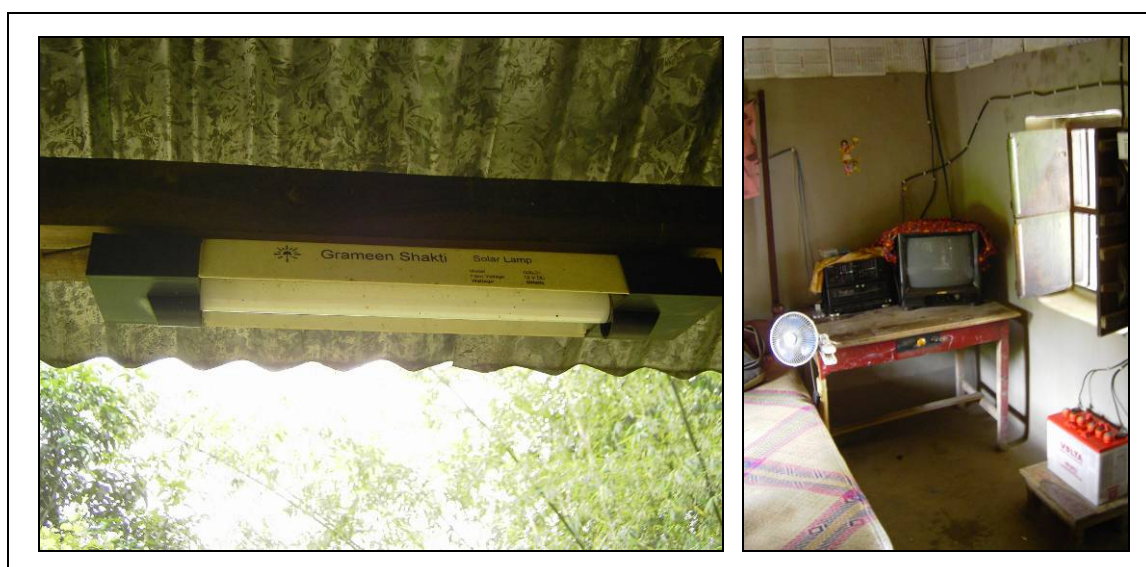
Figure 23: Typical SHS appliances: tube light (left), TV, radio, small fan (right)
