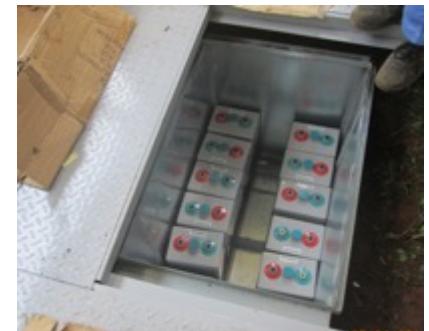
Batteries stored securely inside
