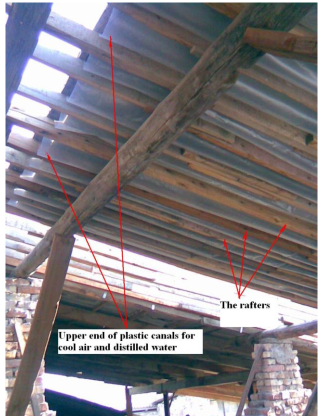
Figure 3: Upper end of the canals for moisturized air
