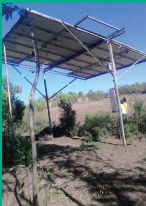
Figure 14: Stolen solar panels at Saremba borehole
