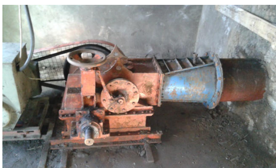
MHP 4104, locally manufactured turbine
