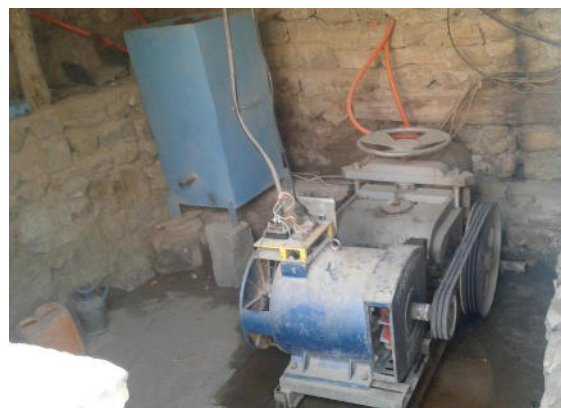
MHP 3106 Often found: mechanically proper turbine-generator assembly but with unprotected generator connections
