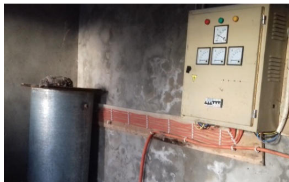
MHP 4126, proper wiring to the ballast tank
