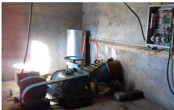
MHP 4135 proper electrical installations but leaking turbine
