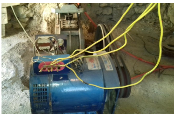
MHP 4034, sub-standard generator wiring
