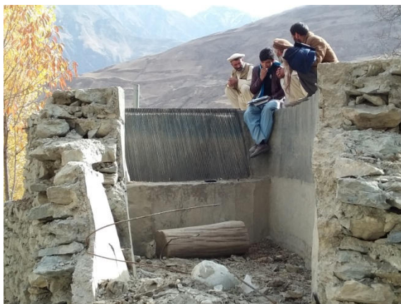
MHP 2014, total flood destruction
