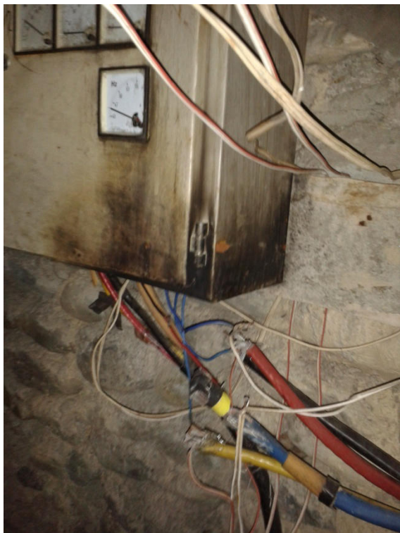
MHP 3007 Non-professionally repaired control panel
