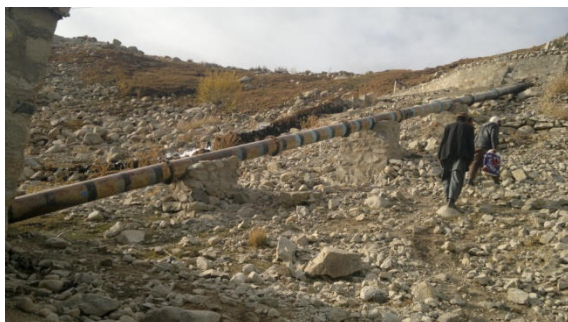
MHP 1031, penstock with supports but without thrust block
