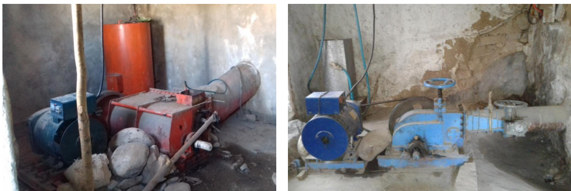
MHP 4124, rocks help improve weak turbine fixation
