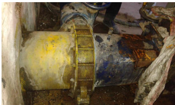
MHP 4157, leaking flange connections
