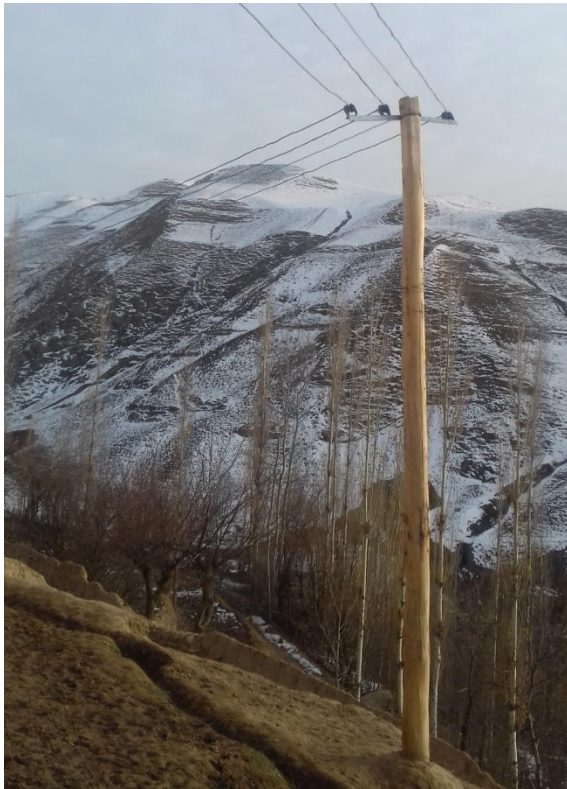
Figure 22 Impressions of local distribution grids and poles used
