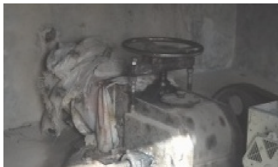
MHP 4129, leaking turbine-penstock connection
