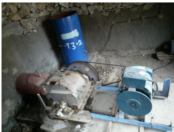
MHP 3044 Low quality turbine without control mechanism
