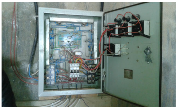
MHP 4104, typical control panel with clearly arranged wiring
