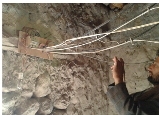
MHP 4039, sub-standard and unsafe electrical wiring
