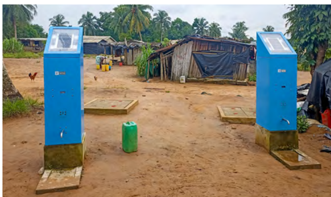
Picture 1: Two automatic standpipes in Tchintchébé
