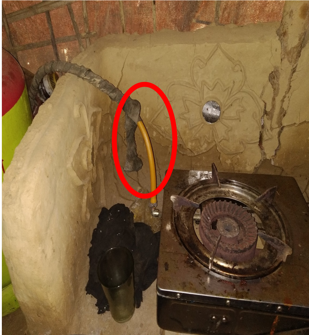
Hose wrapped with cloth
