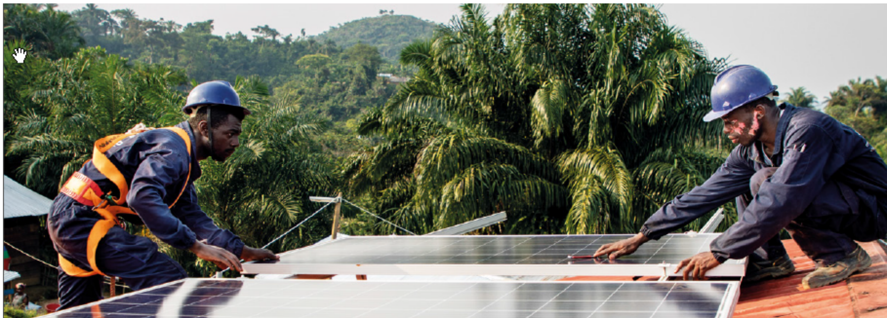
Photovoltaic Systems in Kusisa & Kigulube (Sud Kivu, DRC)
