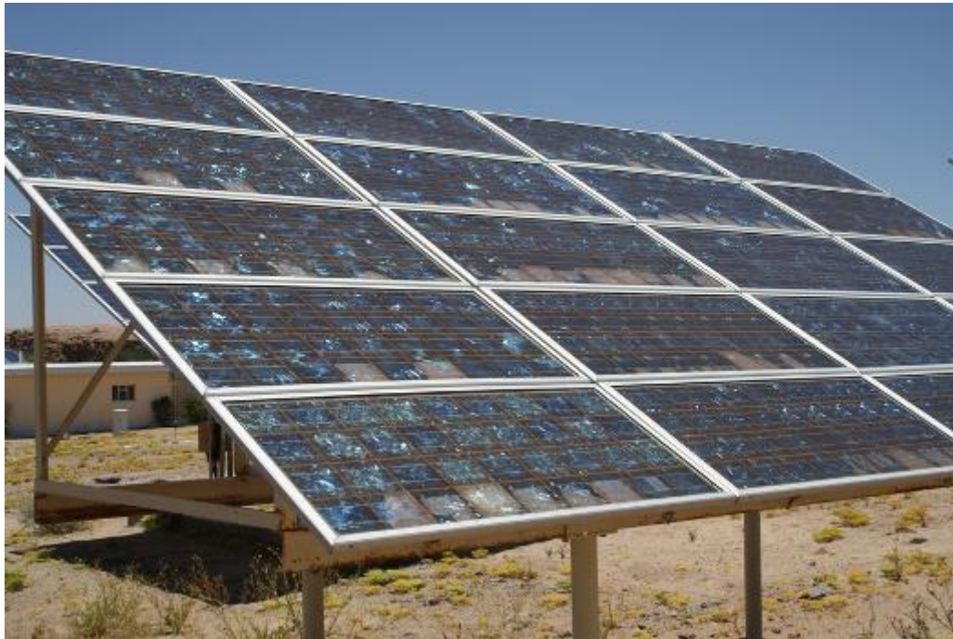
Figure 8: The effect of extreme weather at GTRC and how it is affecting the solar modules
