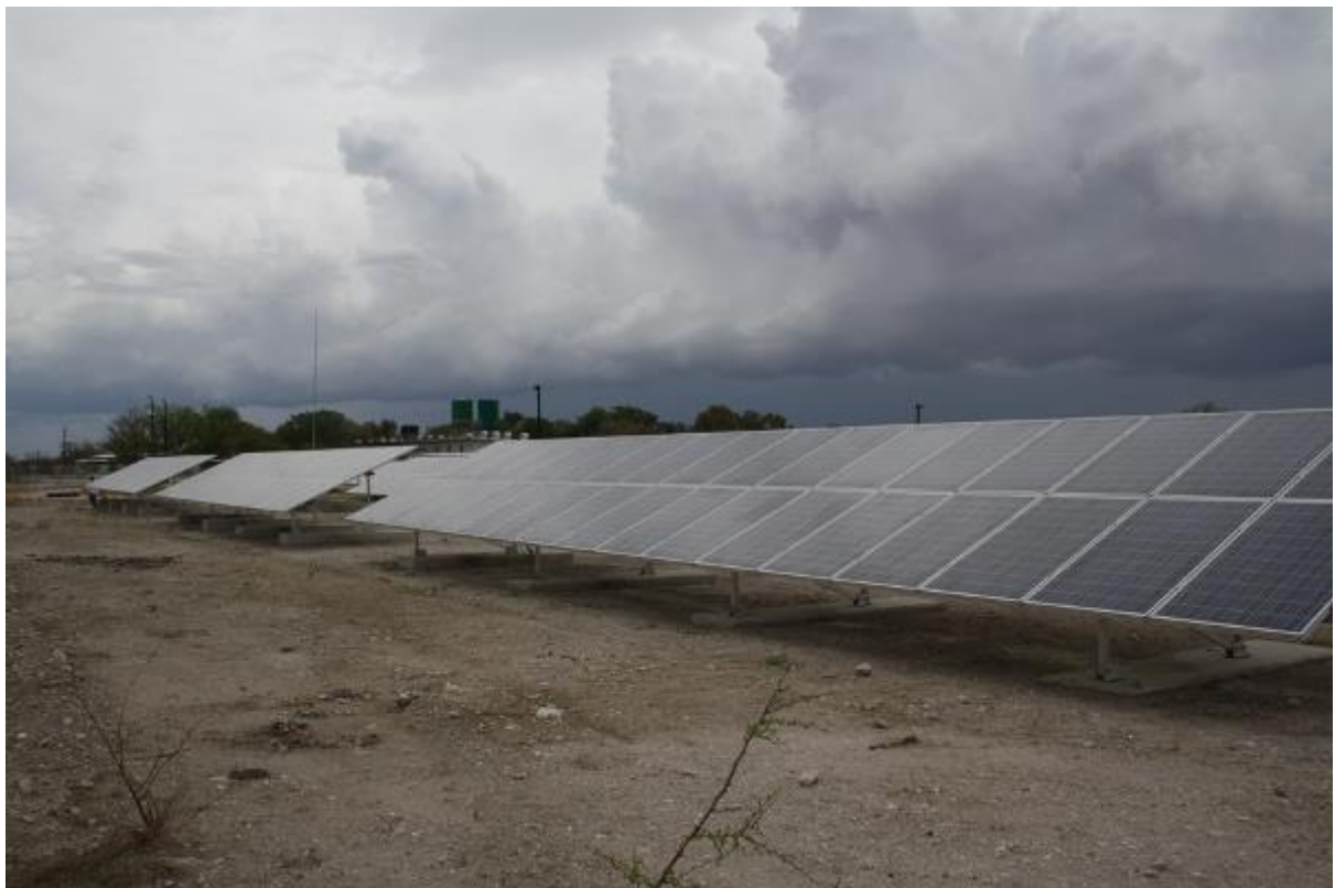
Figure 6: The 202 kWp Tsumkwe Solar Power Plant
