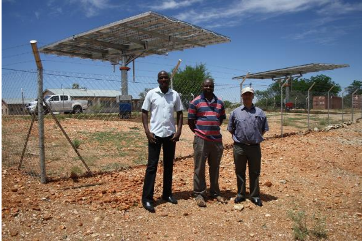
Figure 5: Soitec installed 25 kWp Concentrating Photovoltaic System at Usib Primary School, Rehoboth
