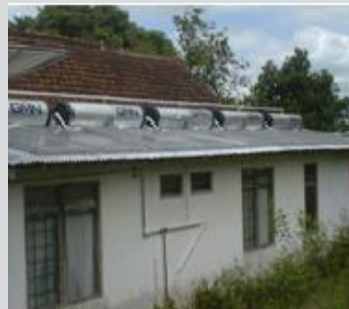
Solar Process Heat
