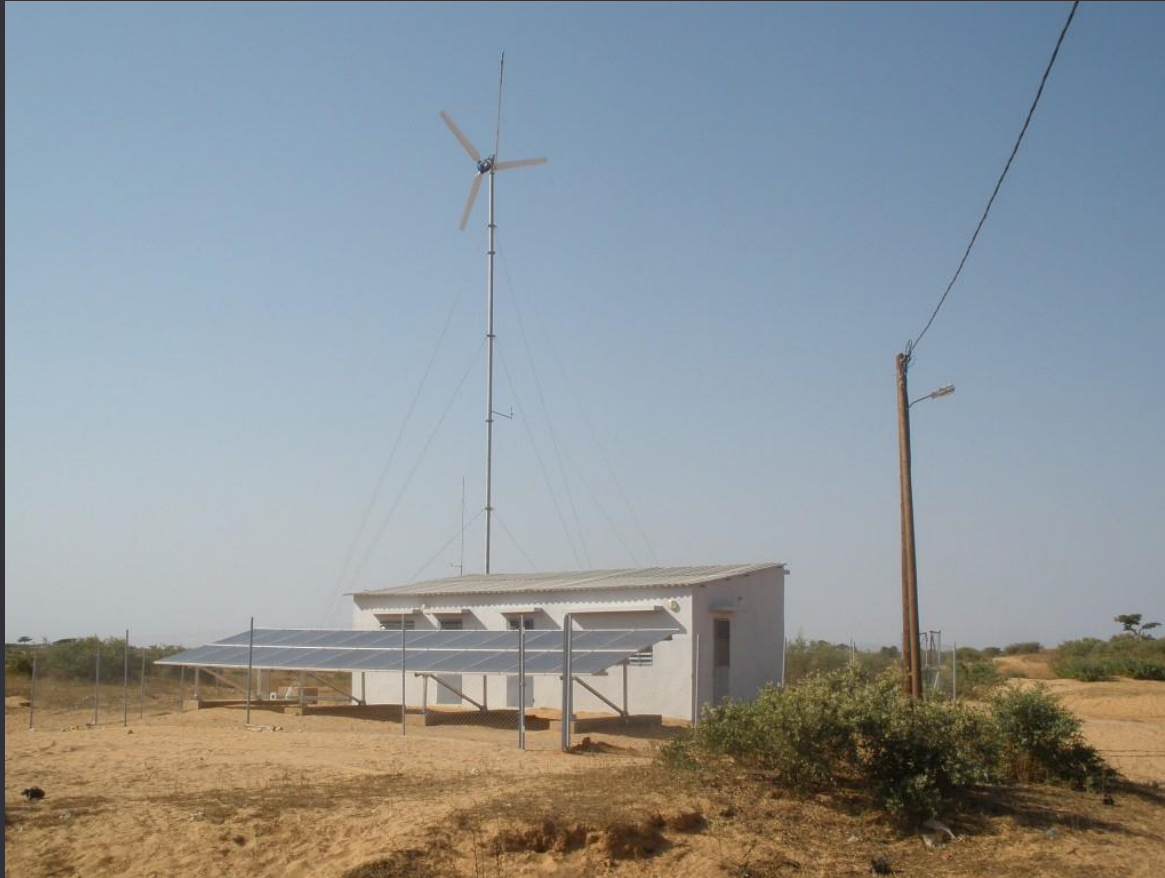
Foto: ENERSA power station; Senegal
