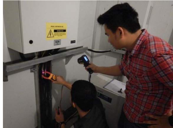
Figure 15 Current measurement on cables detected by infrared camera (thermal imaging)
