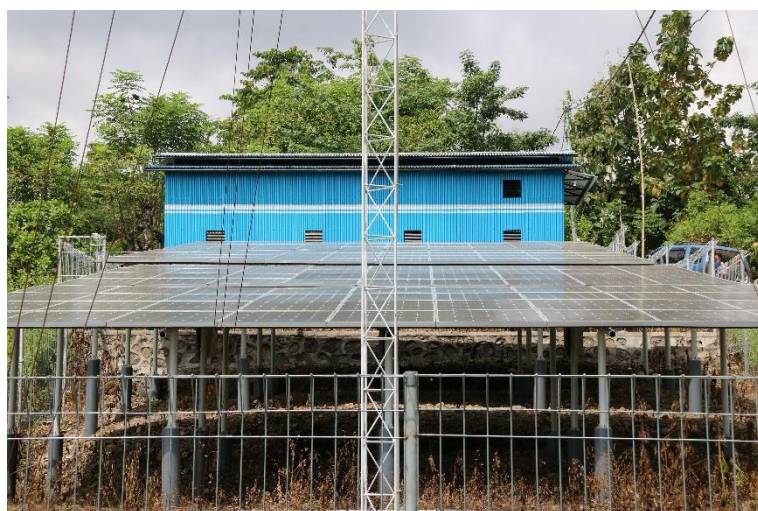
Figure 2 PV mini-grid 30 kWp in Pegadungan, Lombok Utara
