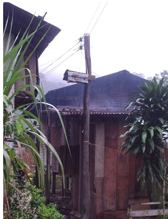
Figure 34. Wooden Transmission post of Buneg MHP
