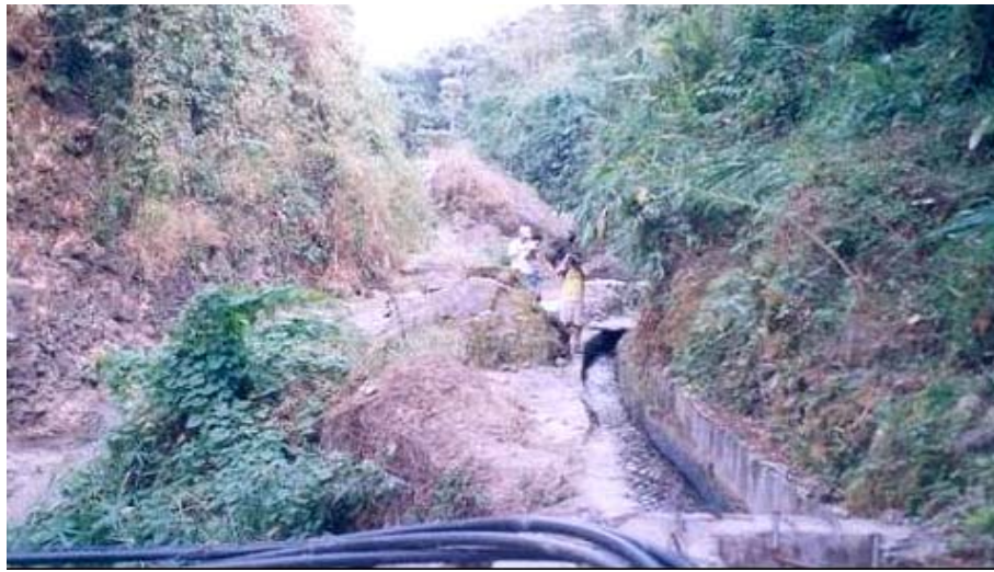
Figure 60. Lon-oy Power Canal
