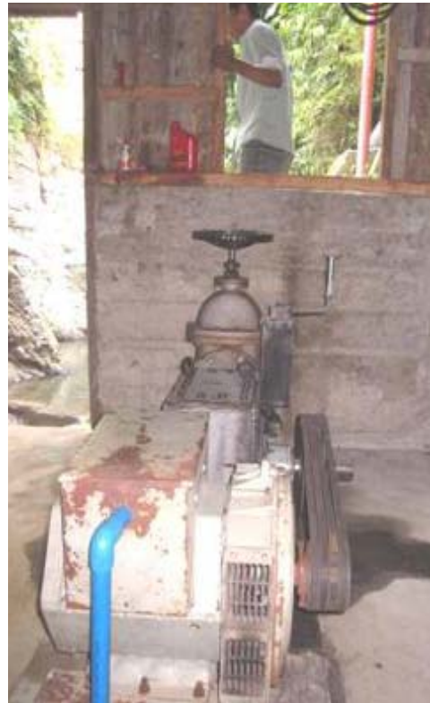
Figure 66. Turbine and generator set configuration inside the Lon-oy Powerhouse
