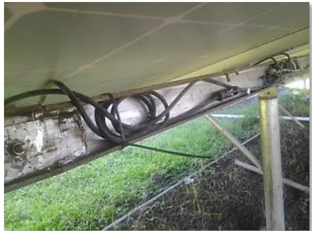
Picture with more than one “object” (in this case: poor wiring, corrosion on steel frame, no conduits and bolts not equal length) reveal more information.
