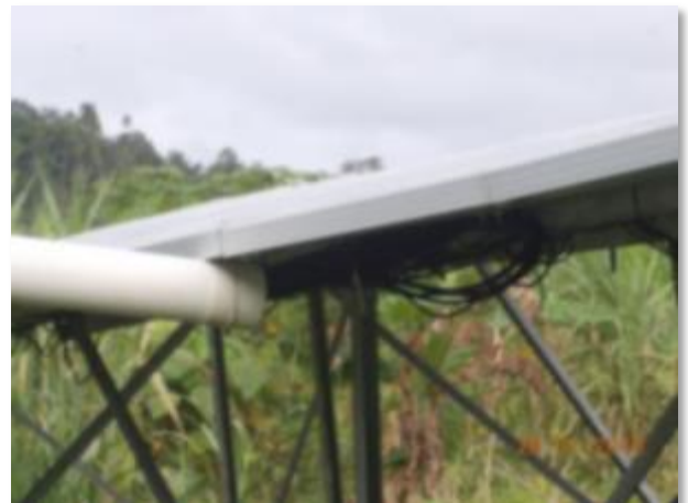
Picture out of focus, too low picture resolution (only 90kB), too close and wrong angle. Angle from below, taken from opposite direction (i.e. showing underside of panels and unsealed conduit opening) would have been better.
