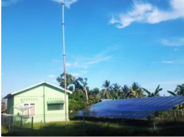
Good overview picture, BUT solar panels cut off. Slight increase of camera distance would have been better.
