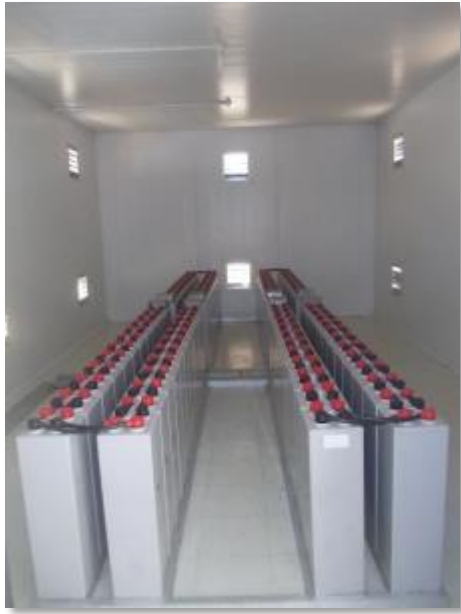
Main object (batteries) very well centred in the picture with correct orientation. Good lighting, sharp focus and picture shows other objects (ventilation openings, neat battery room, conduits).
