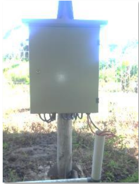
Picture with too much backlight and wrong orientation (landscape orientation from slightly greater distance would show ground conduits and avoid backlight).
