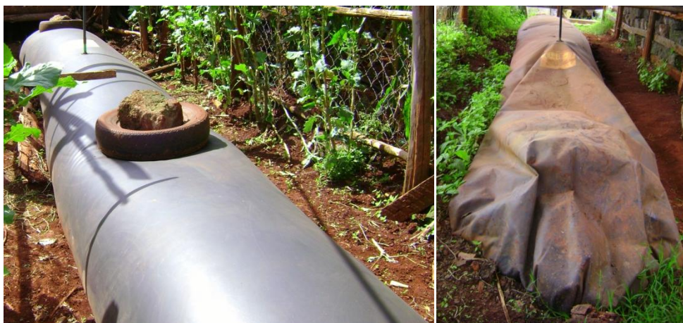
Figure 3: Tight and flat Pioneer digester nearby Nairobi
