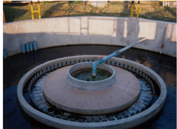
Fig. 2: Pig slaughterhouse Phitsanulok, Thailand: Influent distribution system to UASB reactor (Source: U. Gottschalk, GTZ)
