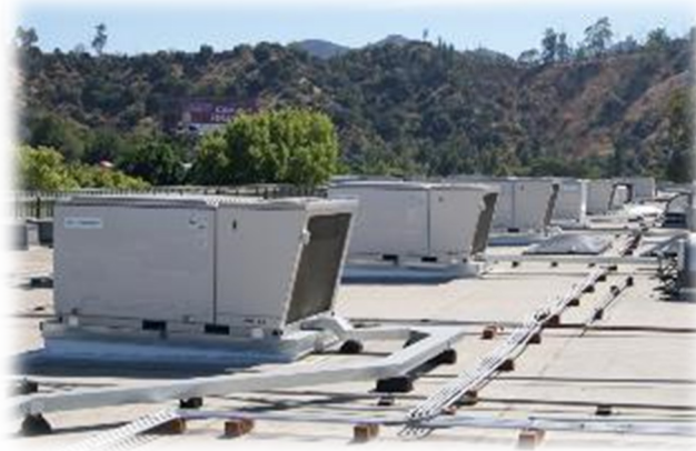
Figure 34. Examples of Thermal Energy Storage Units under Control by GWP
