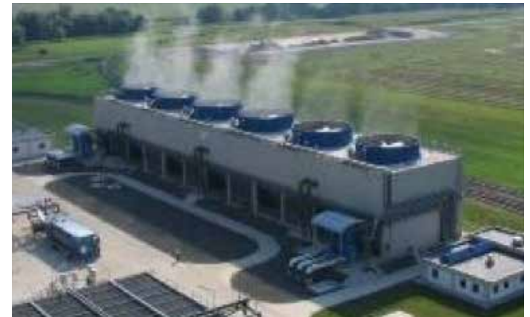
Figure 13: Wet cooling tower, Hungary. GEA, 2004
