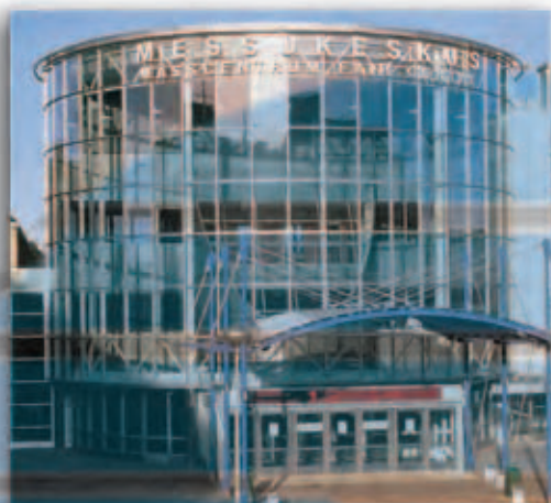
Right: Masscentrum Fair Centre Location: Helsinki, Finland Product: Heat Mirror™ Twin-Coated 88 with Clear Glass
