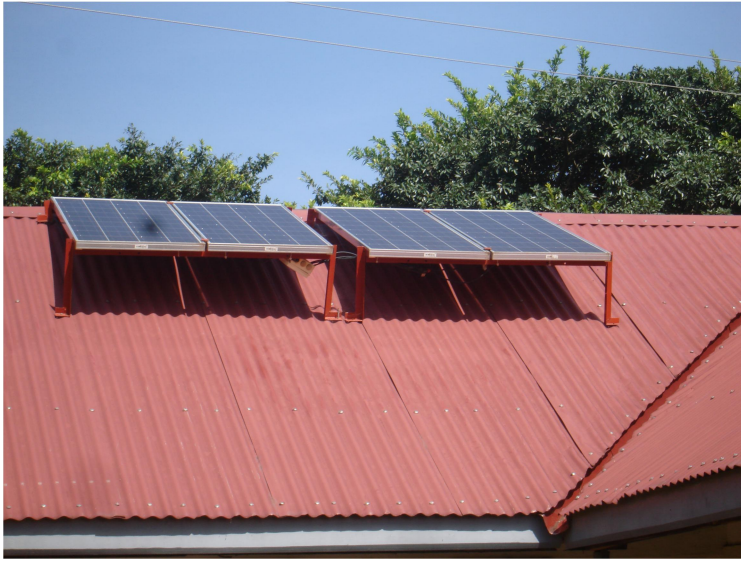
Solar panels mounted on a pitched roof
