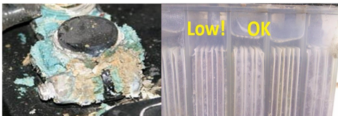
Corroded battery terminal (left); electrolyte level (right)
