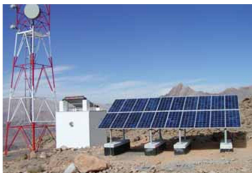
Solar PV system used to power AC loads (only) of a telecommunications tower
