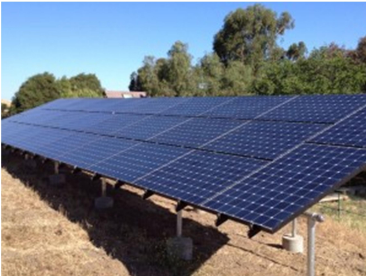
A ground-mounted solar array
