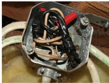
Poor termination and insulation could lead to fires – Courtesy: www.completeepc.co.uk
