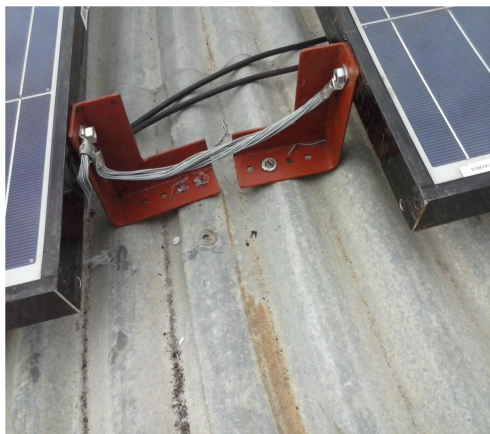
Equipment grounding connection on solar panel frames
