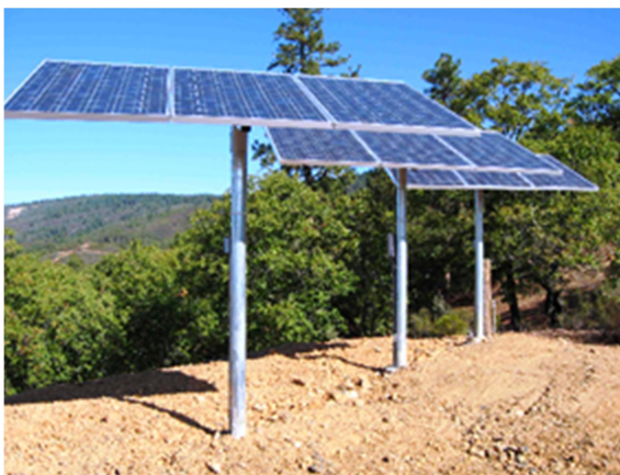
Solar panels mounted on poles
