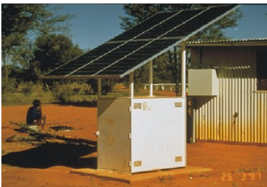
Power supply for lighting in Australia Courtesy: Prof. Dr.-Ing. Habil Ingo Stadler
