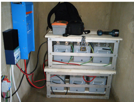
Batteries protected in vented battery box
