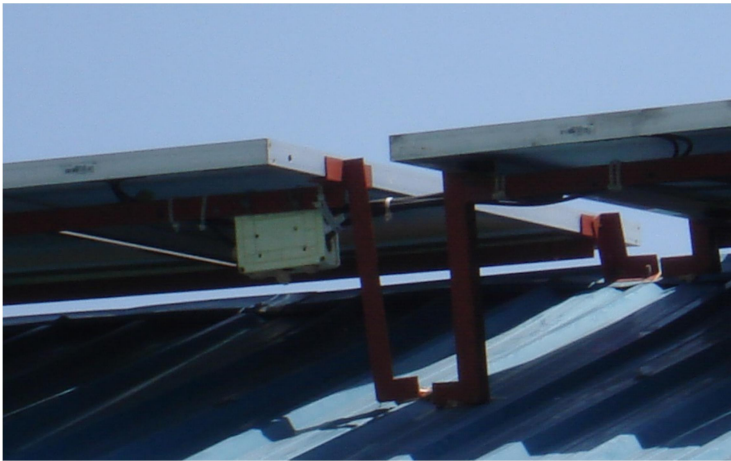
Junction box protected from rain
