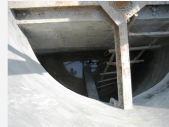
inlet chamber for toilet water
