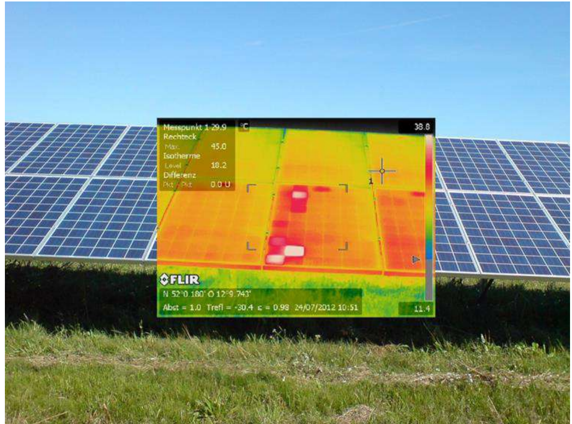
Infrared image of a solar module with several hot spots
