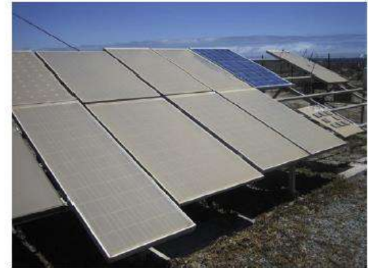
Fig. 3. Heavily soiled modules on the Gran Canaria Island. A manually cleaned module is visible at the top right corner.
