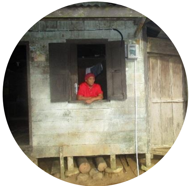
Proper household installation with appropriate grounding and energy limiter protected from the weather. (Source: EnDev ID, GIZ)
