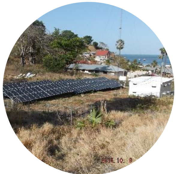
A 30 kWp PV micro-grid in Luang Barat Village, Maluku Barat Daya District providing electricity for 145 households and 8 public facilities.
