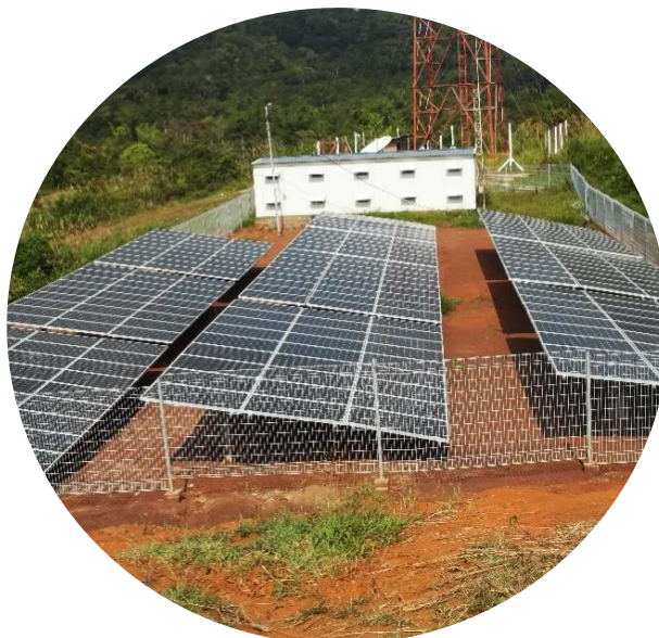
A 50 kWp PV micro-grid in Long Layu Village, Nunukan District, Kalimantan Utara built by KESDM under 2014 budget (Source: EnDev ID, GIZ)
