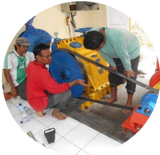
Technical review of micro hydropower. (Source: EnDev ID, GIZ)
