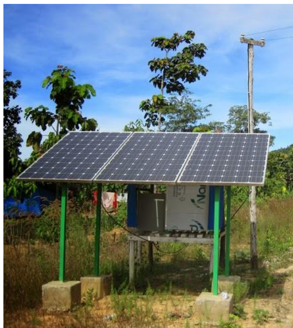
Figure 11: One of nine AC mini-grids installed at Thit Sar Yeik Myaing village in Kayin State.
