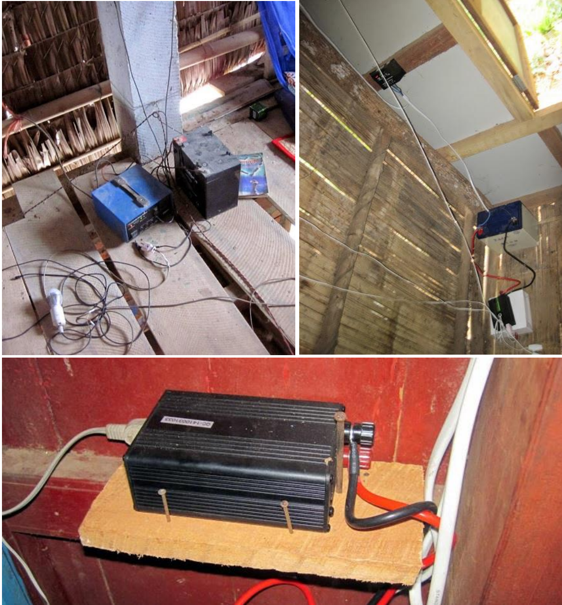
Figure 4: examples of sloppy and hazardous household wiring. In bottom photo notice location of nail immediately next to DC inverter terminals creating a significant fire hazard as these unused wires are connected directly to the battery terminals.
