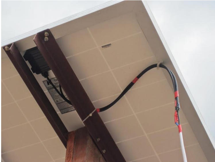
Figure 5: Example of poor splice with wires simply wrapped and taped, also positioned so that it will be soaked in the rainy season.
