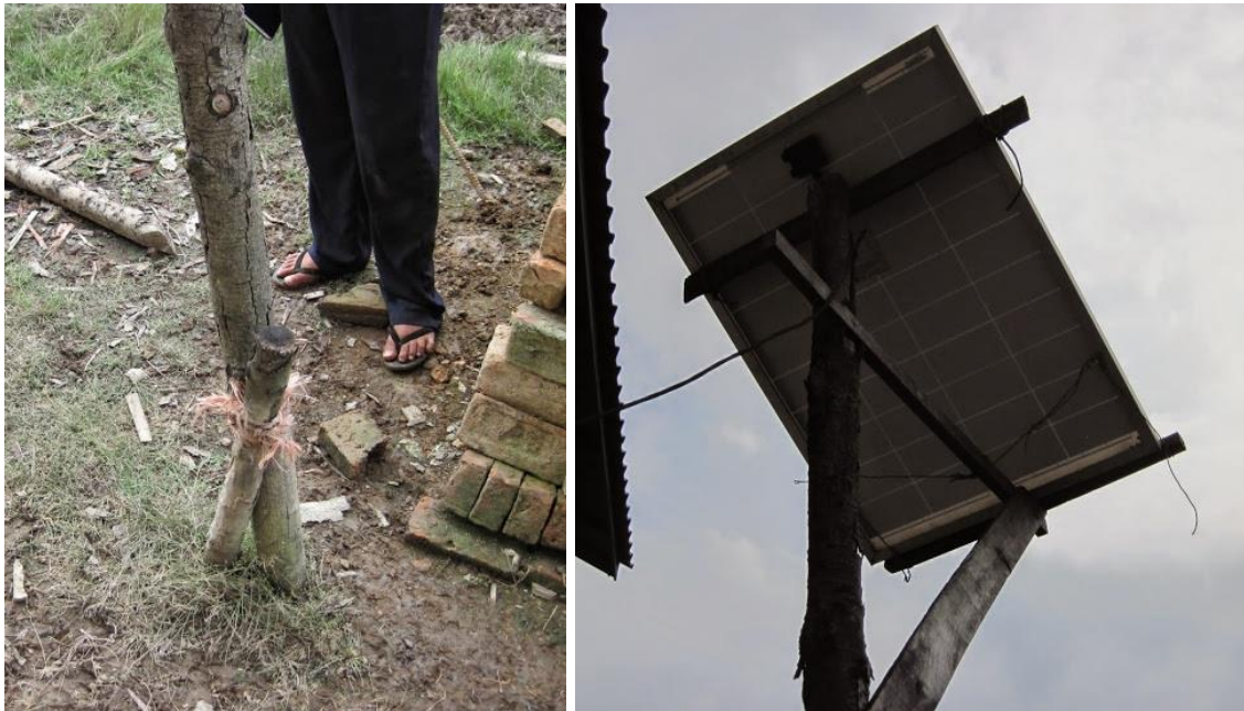
Figure 7: Rot-prone, small diameter poles, flimsy mounting
