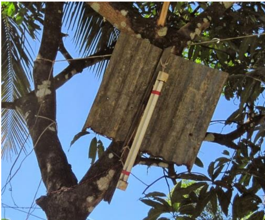
Figure 9: Interior lamp fixtures used in outdoor applications with insufficient rain protection. This
