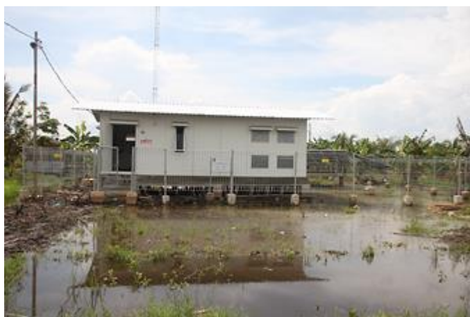
Several PVVP installations are placed in unsuitable sites, which increases risks to technology performance and operator safety.
