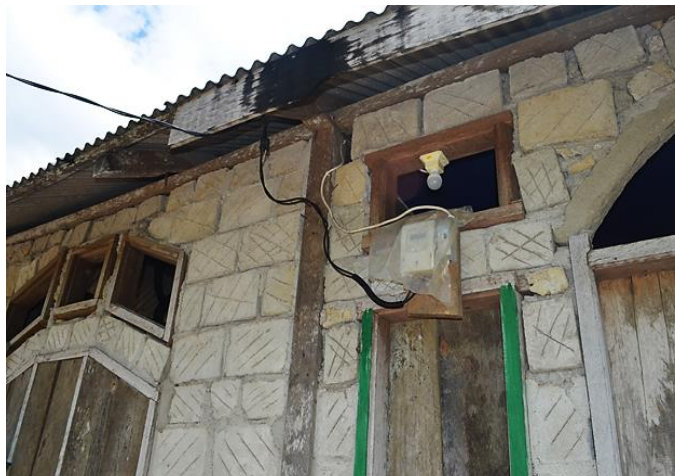
Household installations are still inadequate, often without weather protection, cable conduits and grounding.
