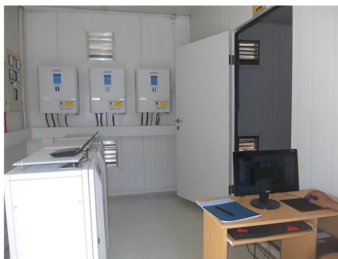
Monitoring hardware (computers) are generally installed, but incorrect configurations provide unreliable data.
