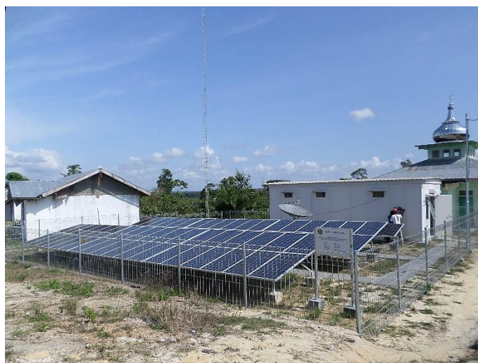
A PVVP installation comprises solar PV modules, a power house for batteries and electronic equipment and a distribution network of cables, connecting all houses.
