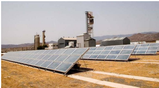
Solar Desalination 1988 High Efficiency 14 stages Plataforma Solar Almeria
