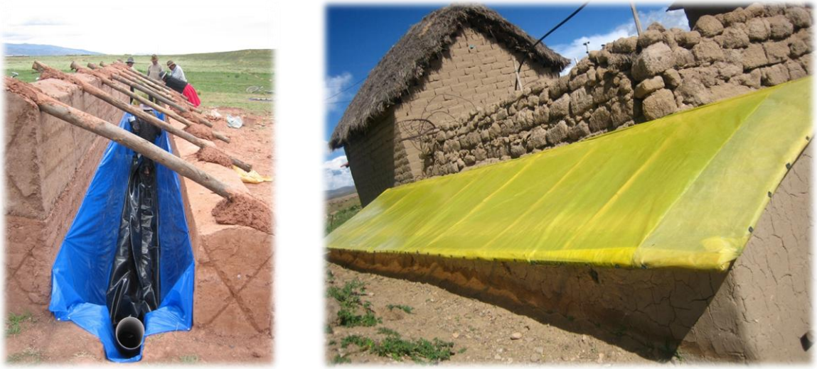
Figure 5: Open and closed trench for a tube digester in the Bolivian Altiplano
