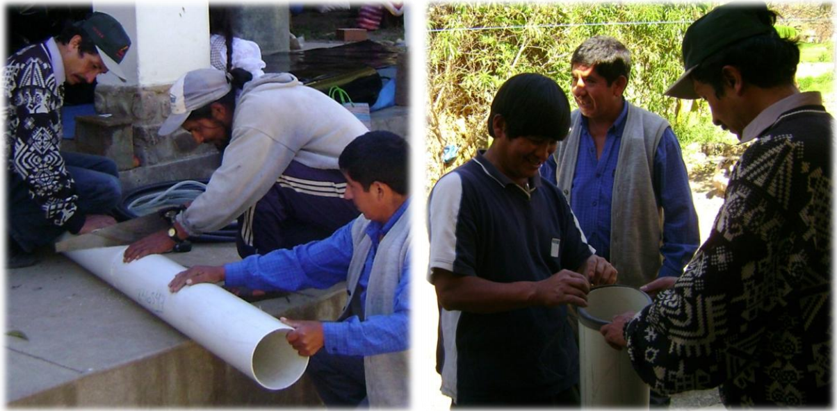
Figure 11: The drainpipe has a length of 4, 0 m normally, so the pipe is cut into pieces of 1, 0 m length. It is to protect the mouths of the in- and outlet pipes, which are introduced inside of the tube digester.
