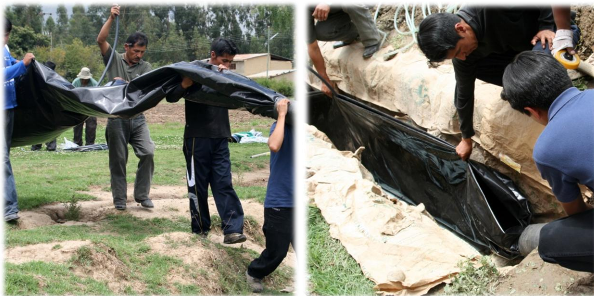
Figure 13: The digester is put very carefully into the trench. The displacement of the tube digester is the most critical situation during the whole installation process.
