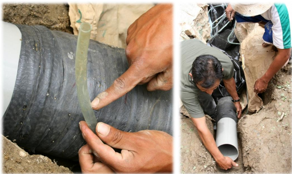
Figure 15: To measure the levels of the outlet, it is easy to use a transparent flexible tube full of water, which indicates the level.
