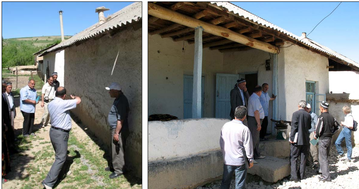
Left – High road side required roof gutter and rainwater evacuation.
