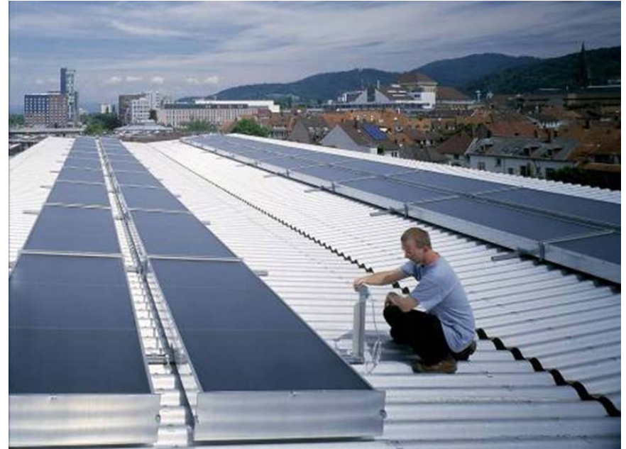
First autonomous solar air-conditioning system in Germany, Chamber of Commerce Upper Rhine
