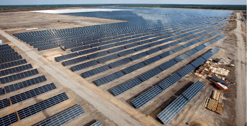
52,79 MW free-field installation, Lieberose (Brandenburg)
