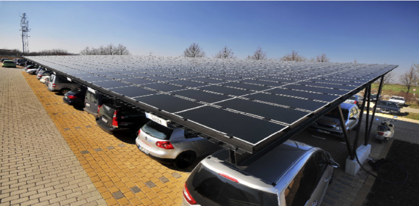
Solar carports at juwi's headquarters in Wörrstadt
