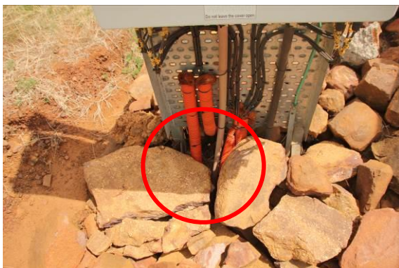
Figure 131: Cable ducts covered with stones
