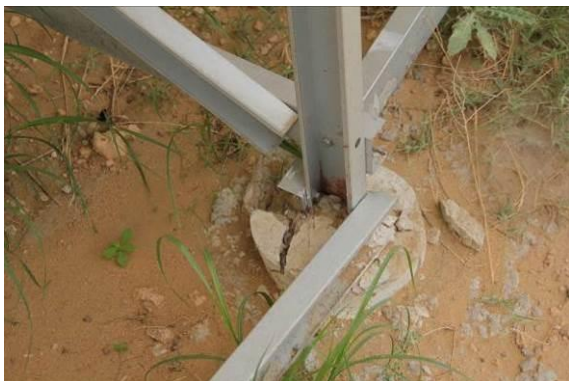
Figure 89: Sporadic damages in the foundation
