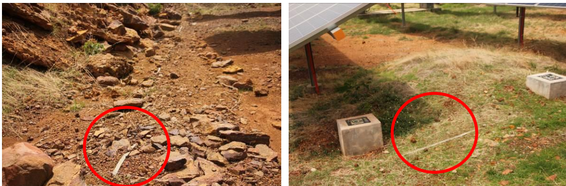
Figure 140: Equipotential bonding conductor not buried
