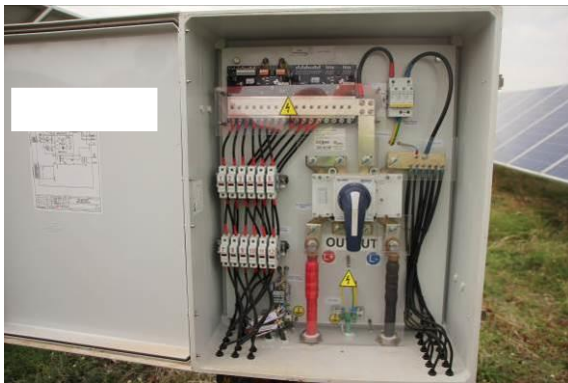
Figure 130: View of the DC combiner box
