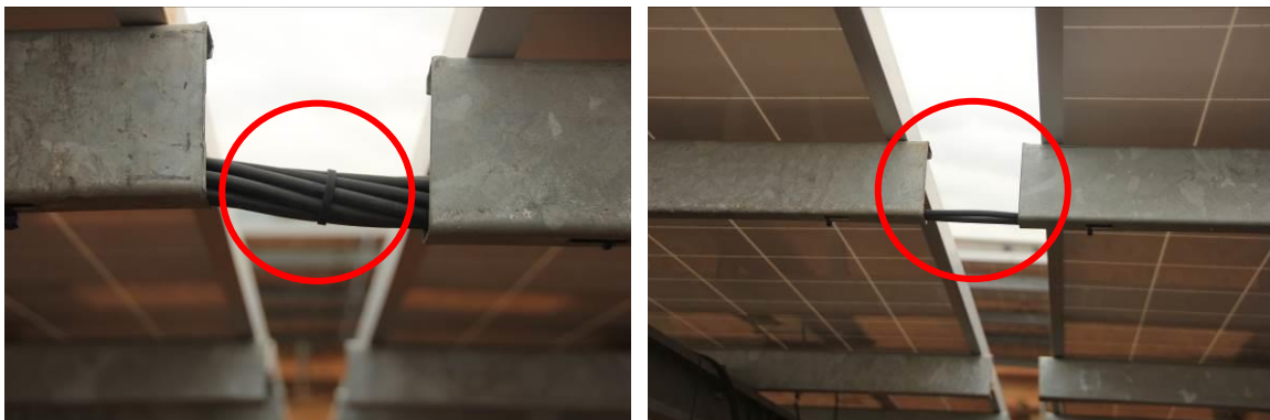
Figure 160: Missing UV protection of the string cables
