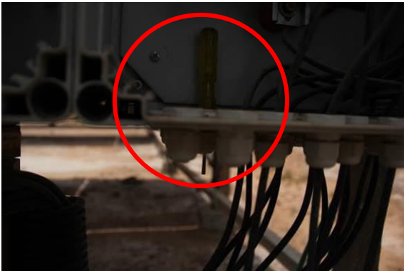
Figure 61: Not sealed cable glands (a screwdriver has been passed through the cable gland to show that it is not properly sealed)
