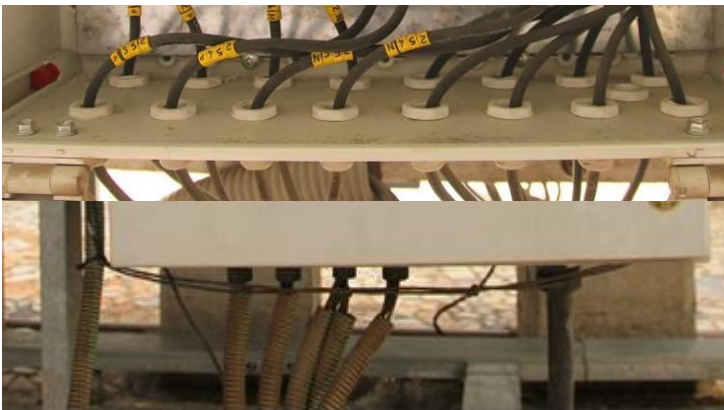
Figure 24: Cable glands of the combiner box
