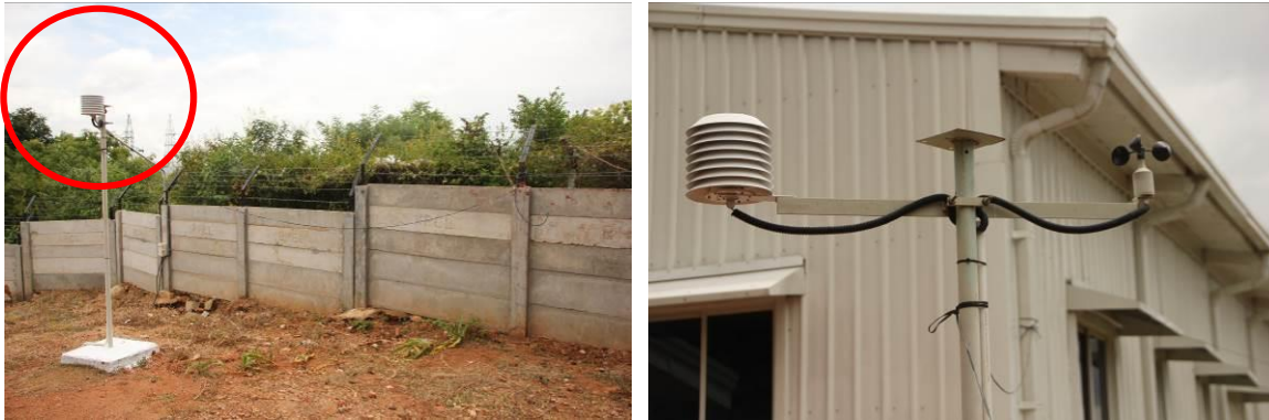
Figure 165: (left) Weather station; (right) Ambient temperature sensor and anemometer
