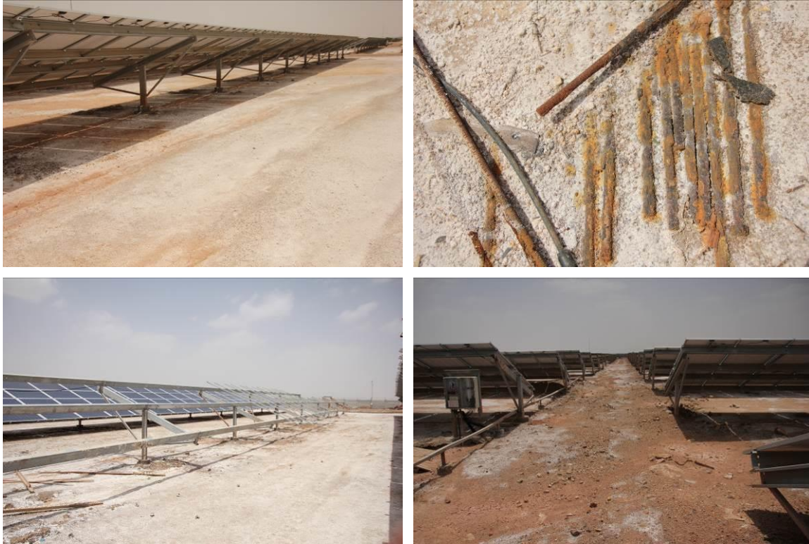
Figure 81: (top and bottom right) Salt presence onsite; (bottom left) Removed modules due to strong winds
