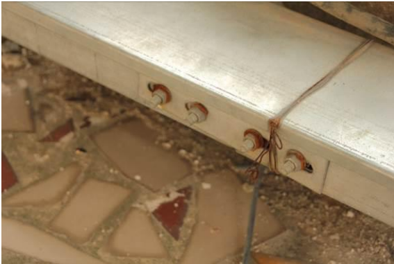
Figure 23: Presence of rust in the mounting structure
