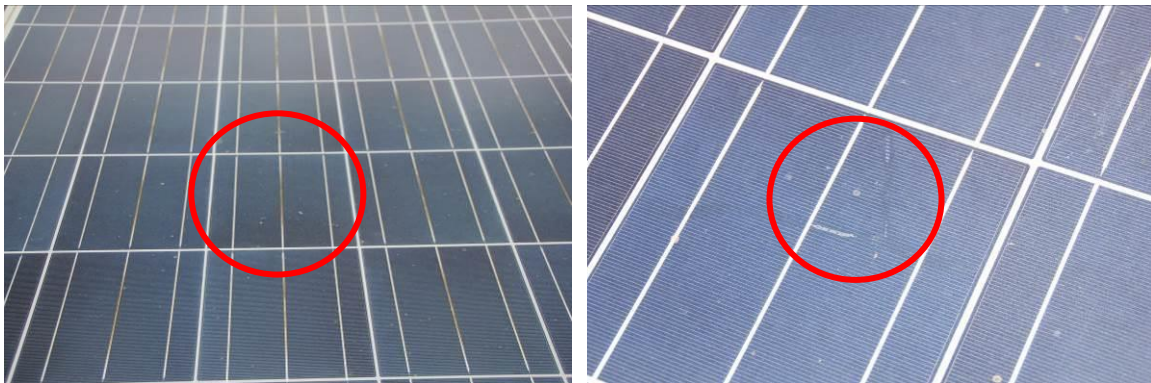
Figure 169: (left) Browning along the busbars; (right) Signs of snail trails
