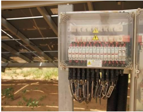
Figure 90: Combiner box view
