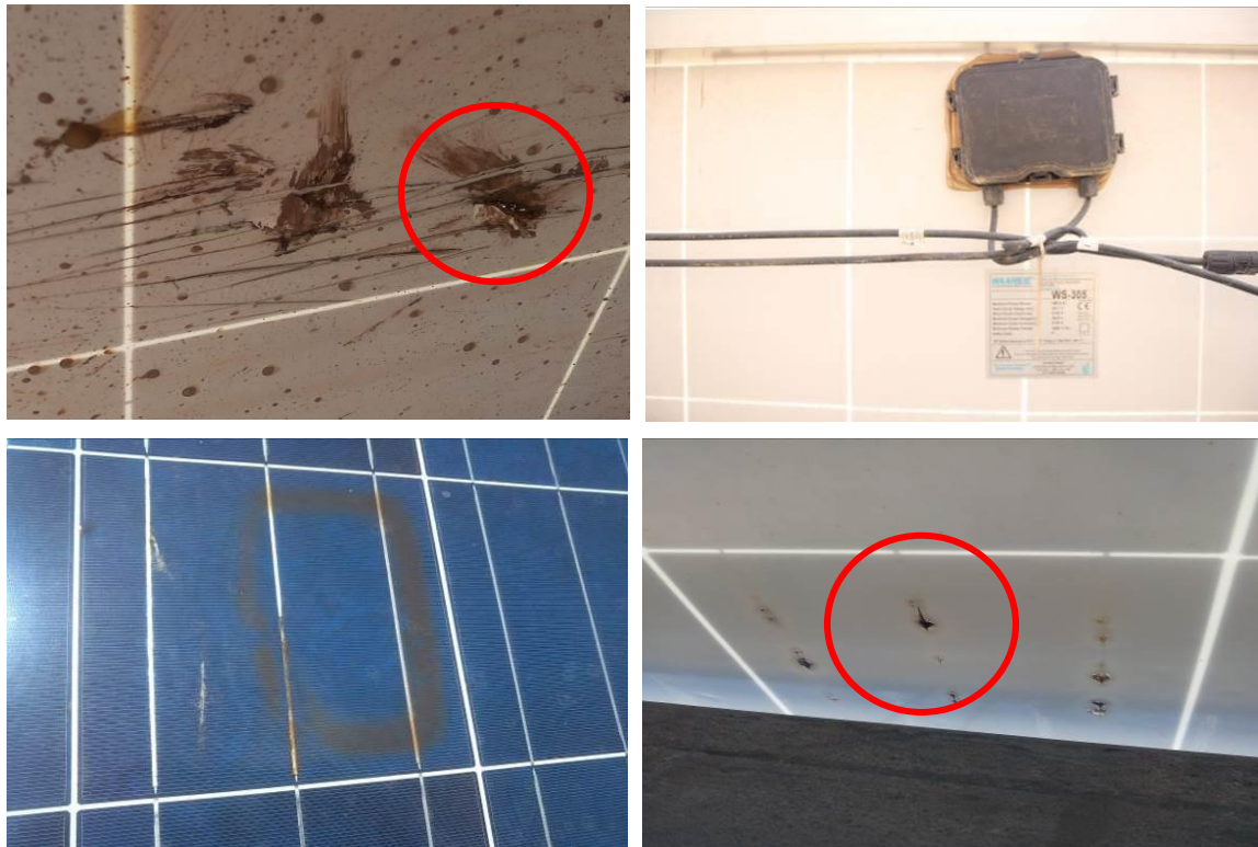
Figure 75: (top left) Scratched module backsheet; (top right) J-box misaligned; (bottom left) Burned cell front; (bottom right) Burned cell
