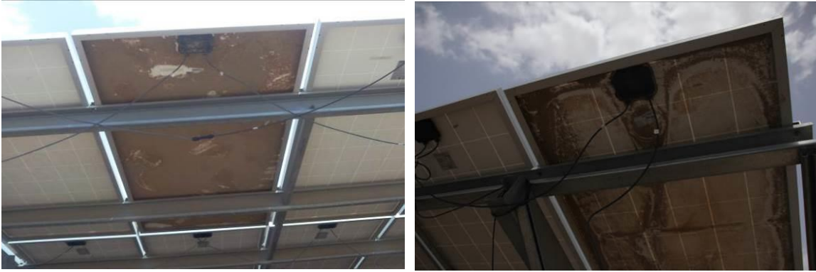
Figure 76: Module backsheet covered with mud
