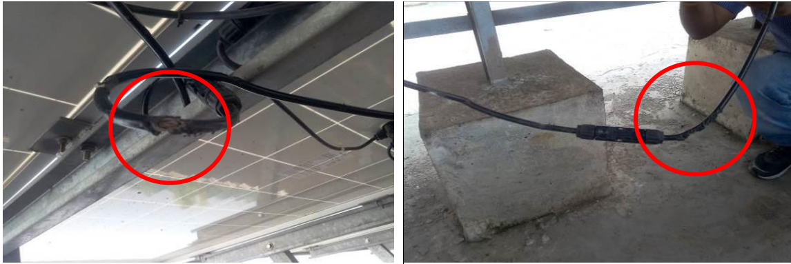
Figure 28: String cables damaged by monkey bites
