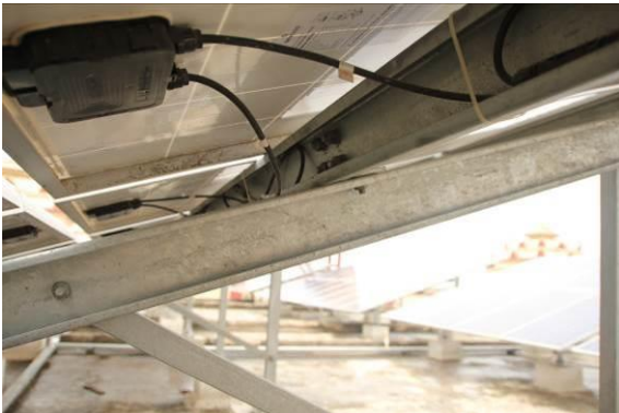
Figure 43: Clean mounting structure surface with no rust
