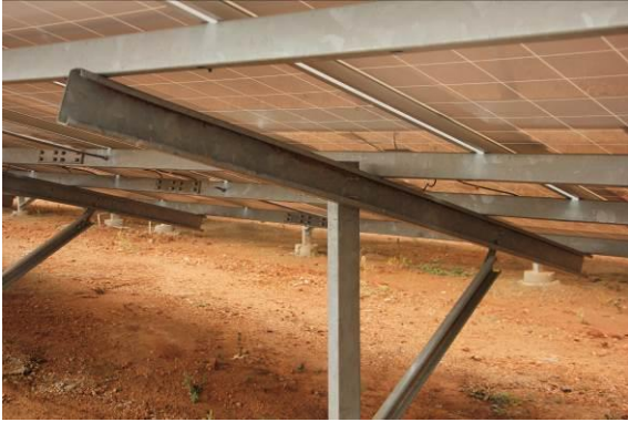
Figure 152: PV modules fixed to the mounting structure
