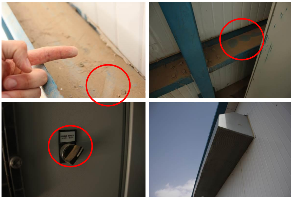
Figure 72: (top and bottom left) Presence of dust inside the PCU; (right) Air inlets of the PCU
