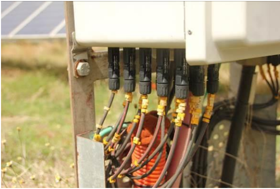
Figure 132: Labelling of the string cables
