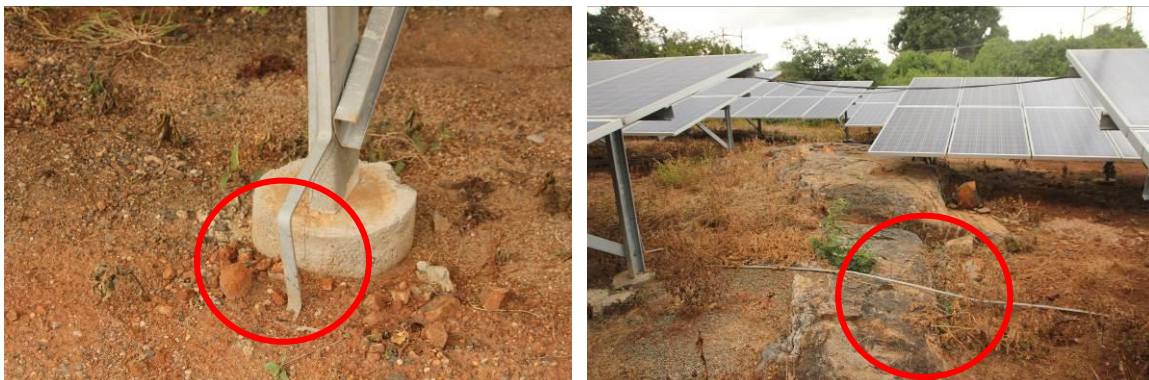
Figure 163: (left) Equipotential bonding conductor; (right) Not buried equipotential bonding conductor
