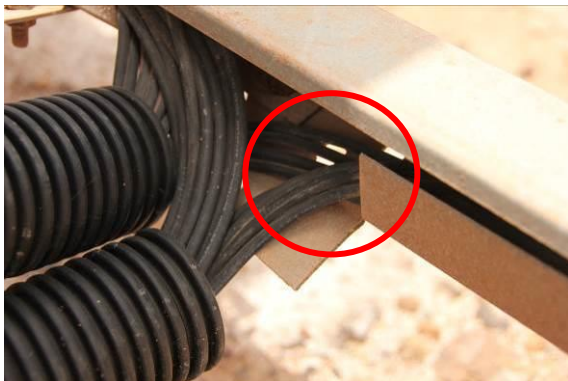
Figure 64: String cables in contact with sharp edges
