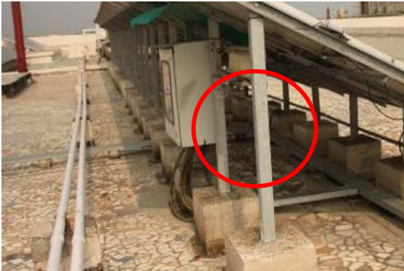
Figure 22: Missing labelling of the module rows
