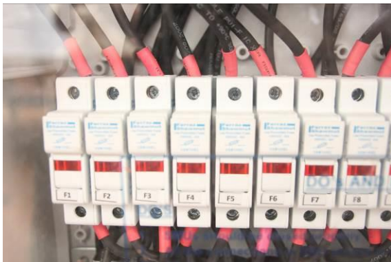
Figure 156: Clean DC combiner box
