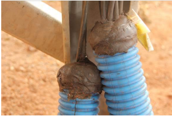
Figure 161: Sealed cable tubes
