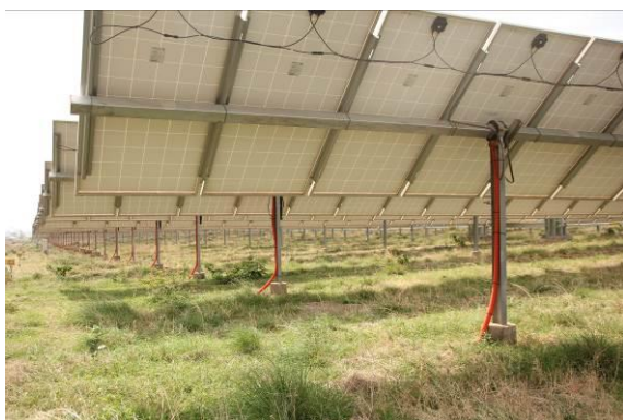
Figure 137: Cable pipes used for the string cable routing
