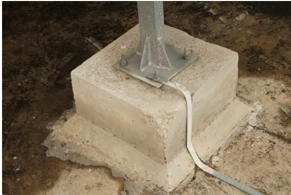
Figure 50: Equipotential bonding system conductor
