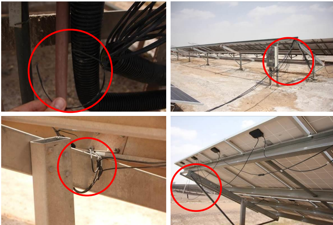
Figure 67: Improper cable fixation of the string cables
