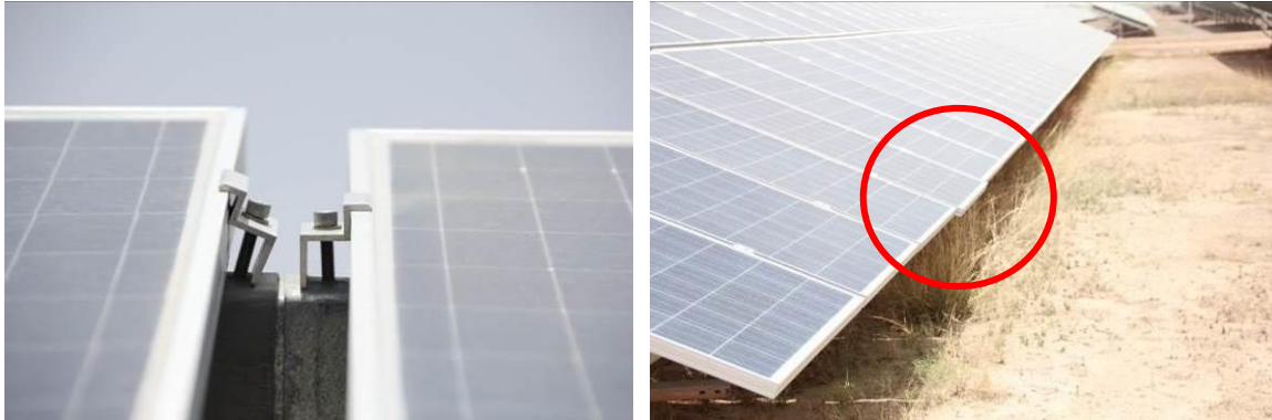
Figure 58: Improper module fixation
