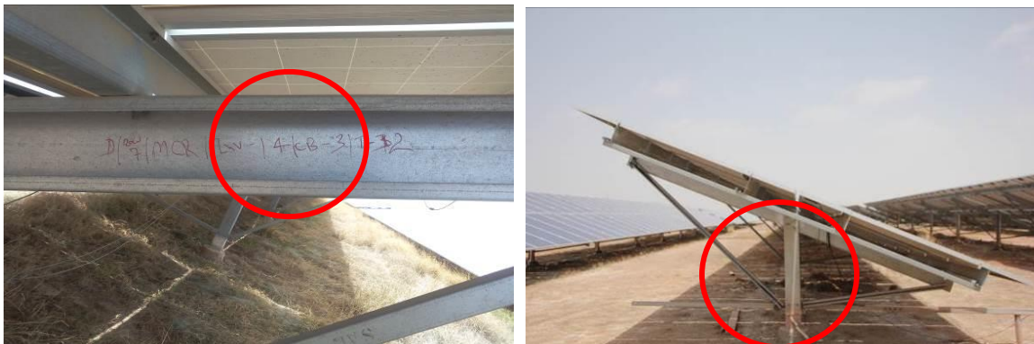
Figure 59: Improper row labelling
