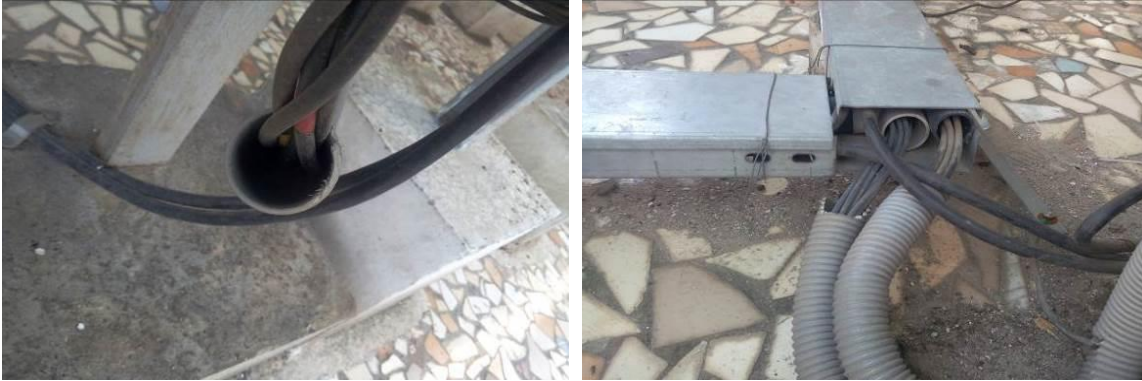
Figure 34: Non sealed cable tubes
