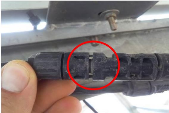
Figure 31: PV module connectors not properly closed
