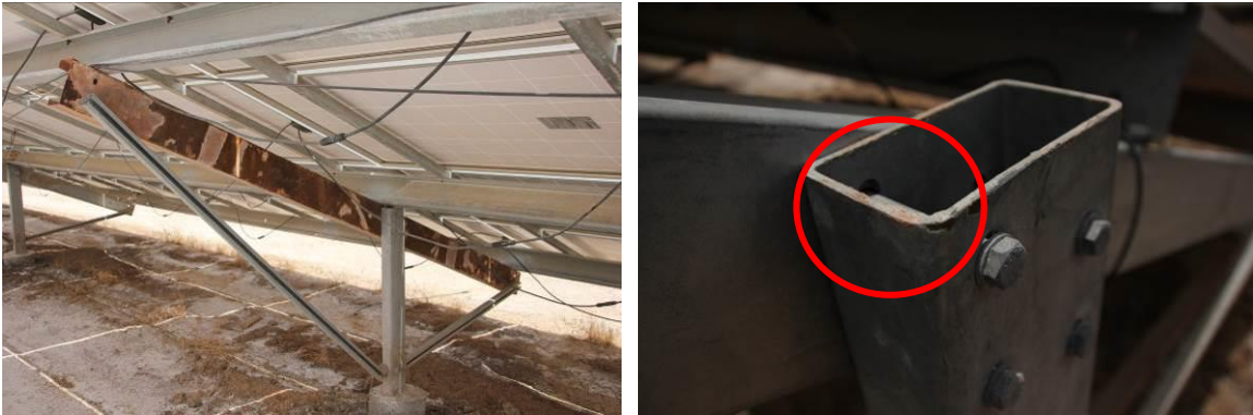
Figure 60: Mounting structure affected by rust due to the salty environment
