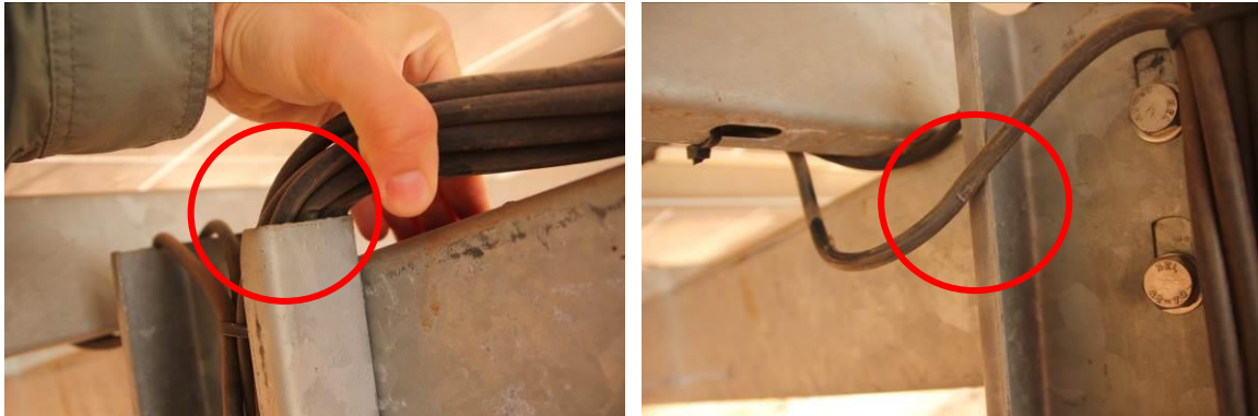
Figure 158: String cables in contact with sharp edges
