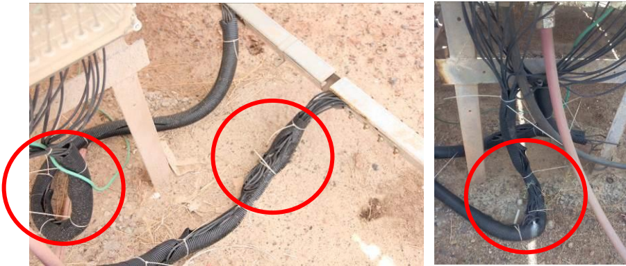
Figure 71: Degraded cable pipes due to outdoor exposure
