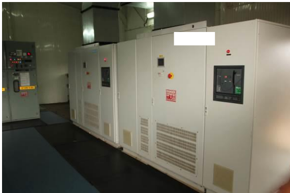
Figure 162: View of the central inverter
