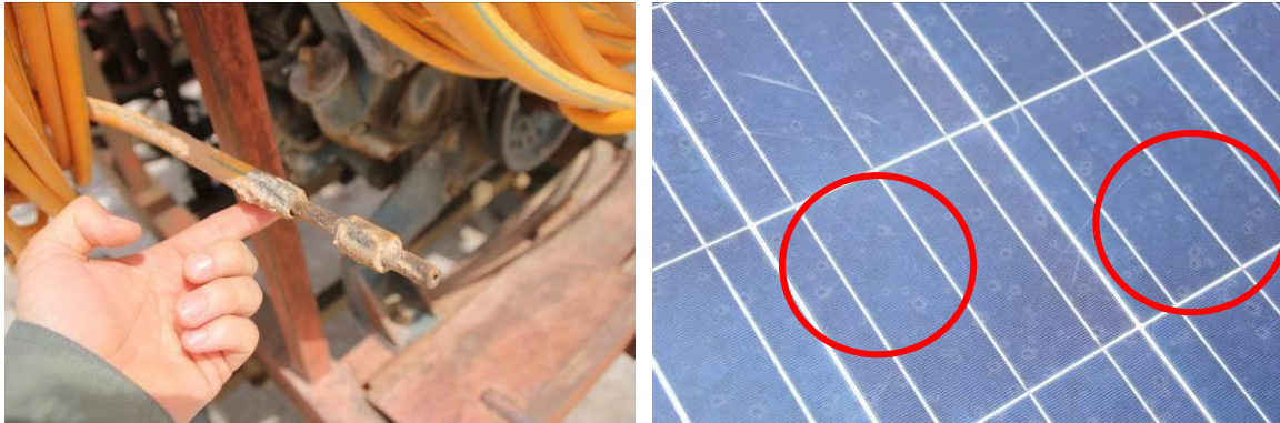
Figure 82: (top and bottom left) Module cleaning system; (bottom left) Dust and soil attracted by water drops
