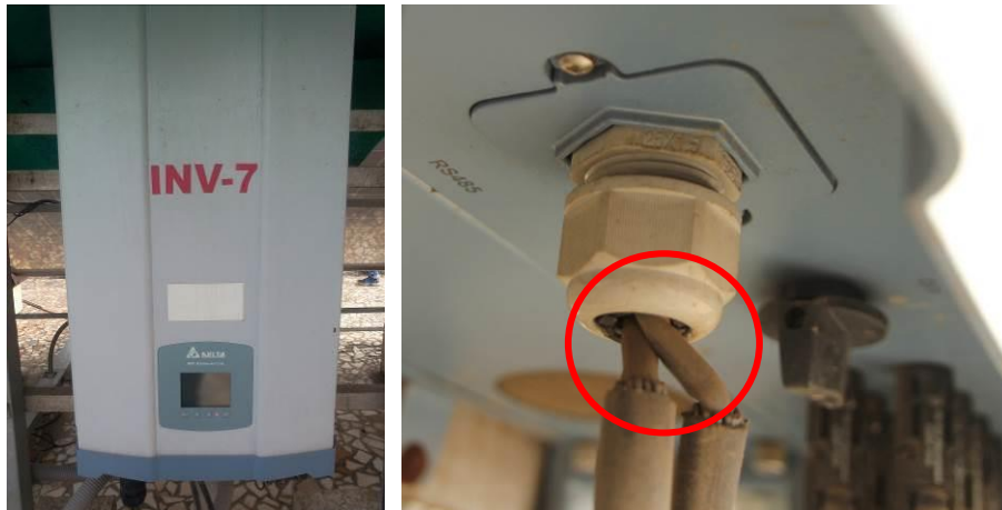
Figure 36: (left) String inverter; (right) Unprotected interface between communication cables and inverter housing
