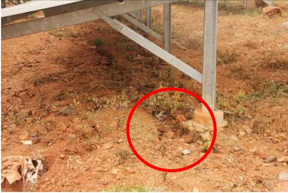
Figure 176: Signs of erosion
