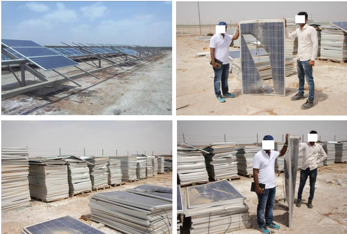
Figure 56: Damaged modules due to strong winds
