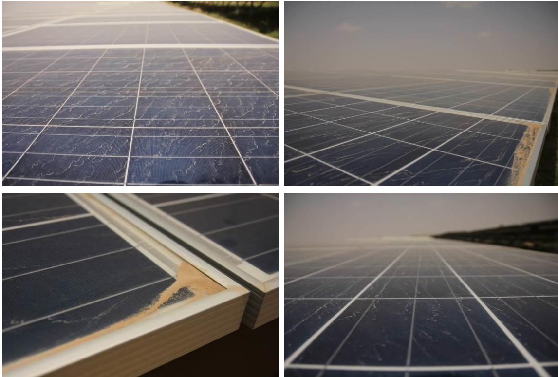
Figure 115: Dust accumulated on the remaining water after the cleaning process
