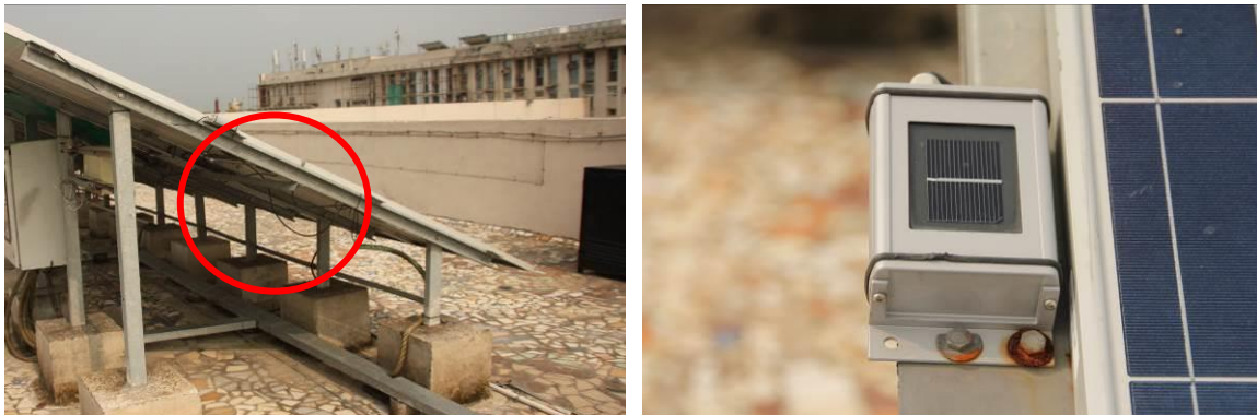
Figure 38: (left) Not protected communication cable; (right) Irradiation sensor installed onsite
