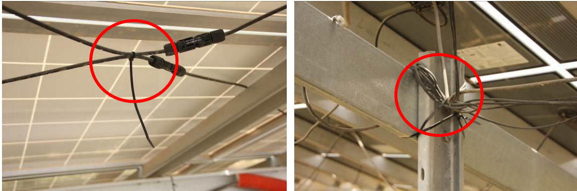
Figure 95: Improper cable fixation
