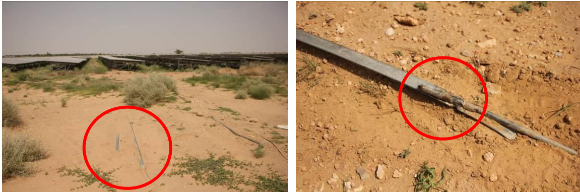
Figure 101: Not buried equipotential bonding conductor
