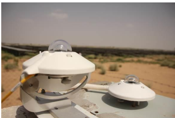
Figure 105: Pyranometers on the horizontal and tilted surface
