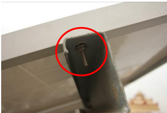
Figure 41: Loose fixation of the PV modules to the cross beam
