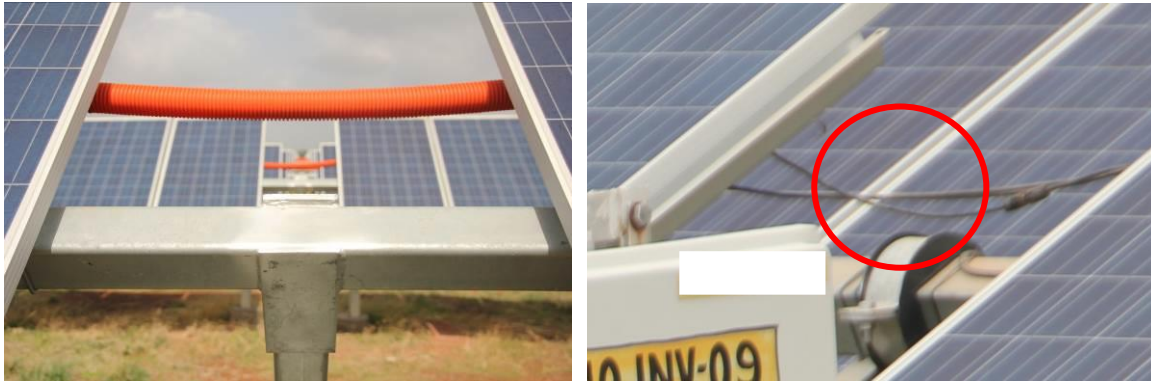
Figure 135: (left) UV protection of the string cables; (right) Missing UV protection of the string cables
