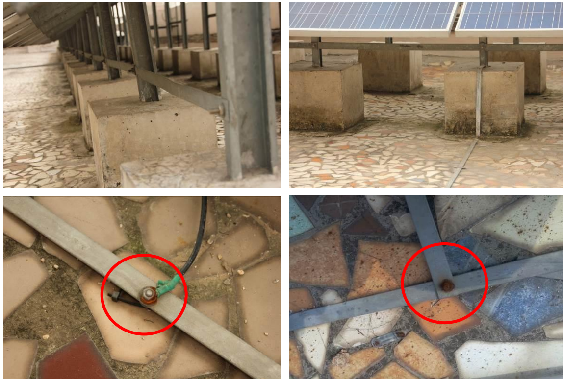
Figure 37: (Top) Equipotential bonding system installed onsite; (bottom) Rust in the equipotential bonding system
