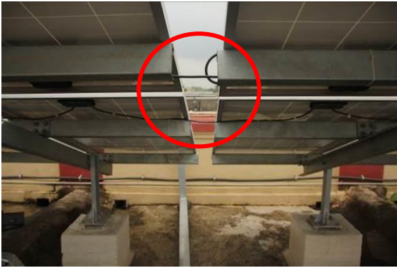
Figure 47: Missing UV protection of the string cables
