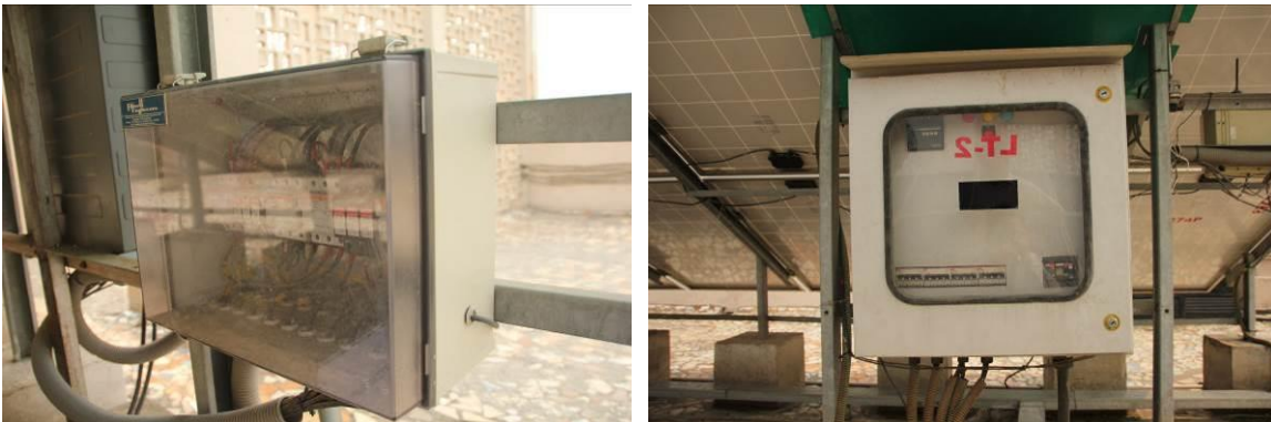
Figure 27: (left) Missing labelling of the DC combiner box; (right) Labelled AC combiner boxes
