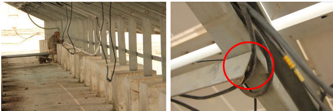
Figure 29: (left) Monkeys present on site; (right) String cables in contact with sharp edges
