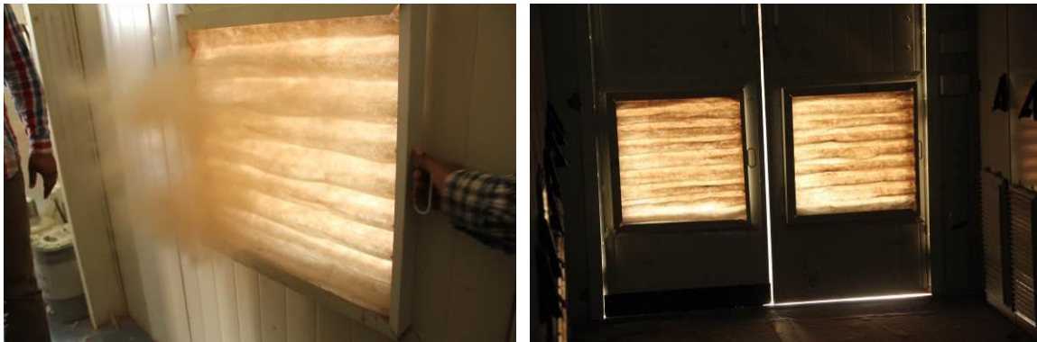
Figure 99: Dirty filters due to dust accumulation
