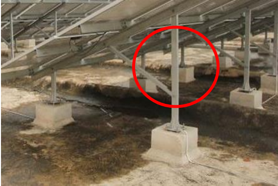
Figure 42: Missing labelling of the module rows
