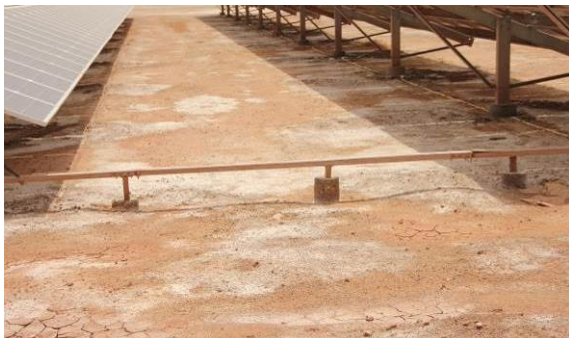
Figure 83: Cable routing system disturbing the access by car to the interrow space
