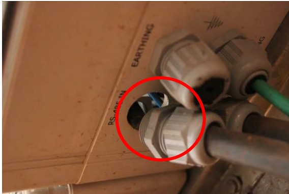
Figure 155: Open cable glands in the DC combiner box
