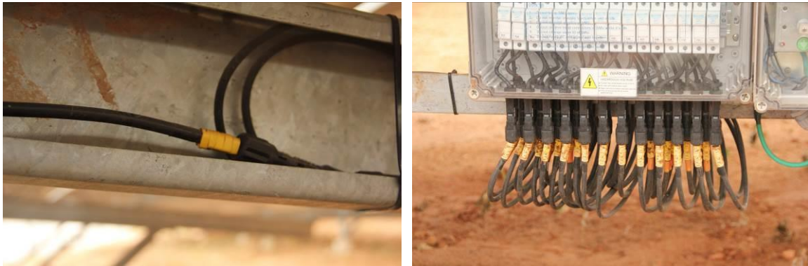
Figure 159: Labelling of the string cables
