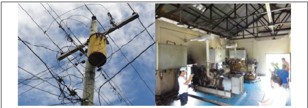
Photo 1: Local power distribution and generation facilities on Carabao Island
