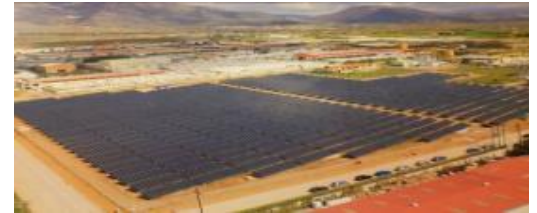
PV-free-field installation Drama, Greece
