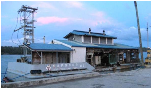
Mobile diesel power generation plant – Siquijor Island, Philippines (Bertheau, 2013).
