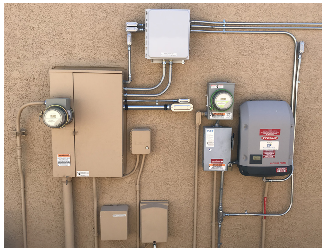
Figure 7 – Example battery energy storage system (outdoor) installation, including power monitoring equipment (top middle of photograph)
