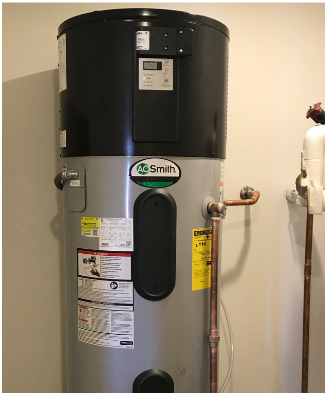
Figure 5 – Example grid-interactive water heater (indoor) installation
