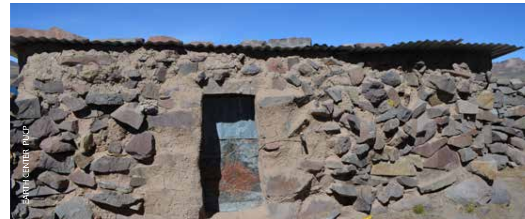
The research looks to improve the architectural conditions of homes in rural Andean regions.
